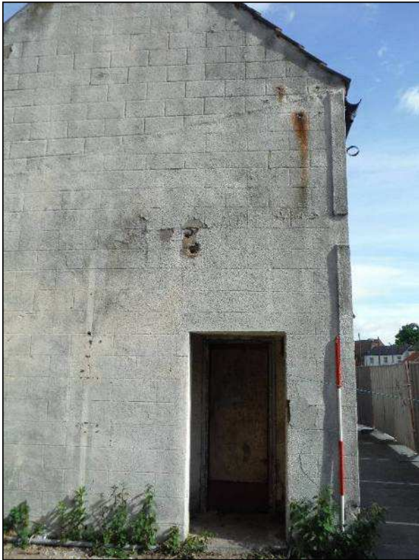
Plate 3 (Shot 20): South elevation showing marks in the render, looking north (2m scale)
