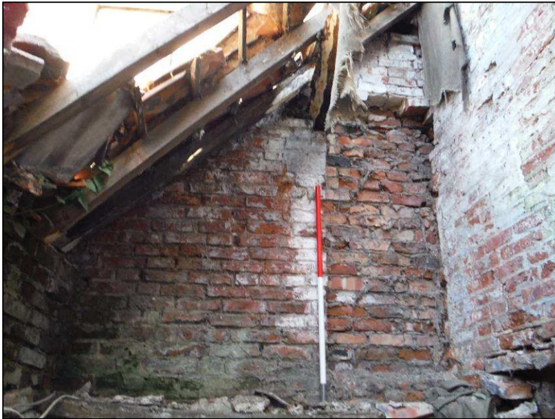
Plate 29 (Shot 81): Blocked door leading from the first floor of the lean-to extension into the main part of the house, looking north (1m scale)
