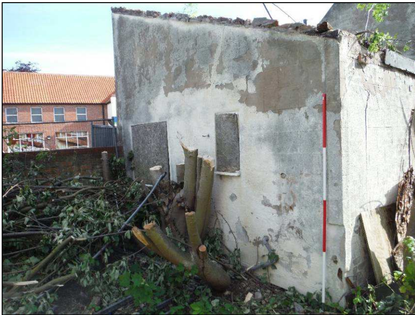
Plate 6 (Shot 14): Single storey extension projecting west from the original building, looking northeast (2m scale).
