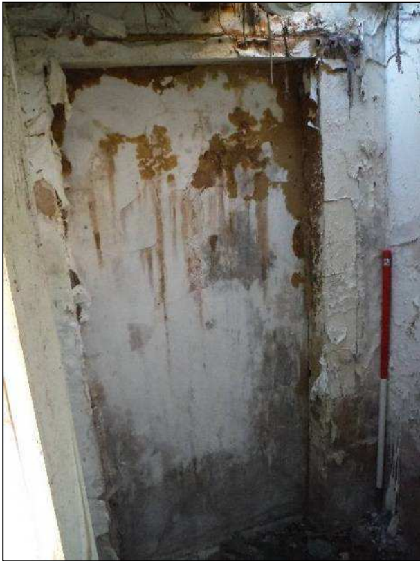
Plate 18 (Shot 44): Blocked door in the southern elevation in the shower room, looking southwest (1m scale)
