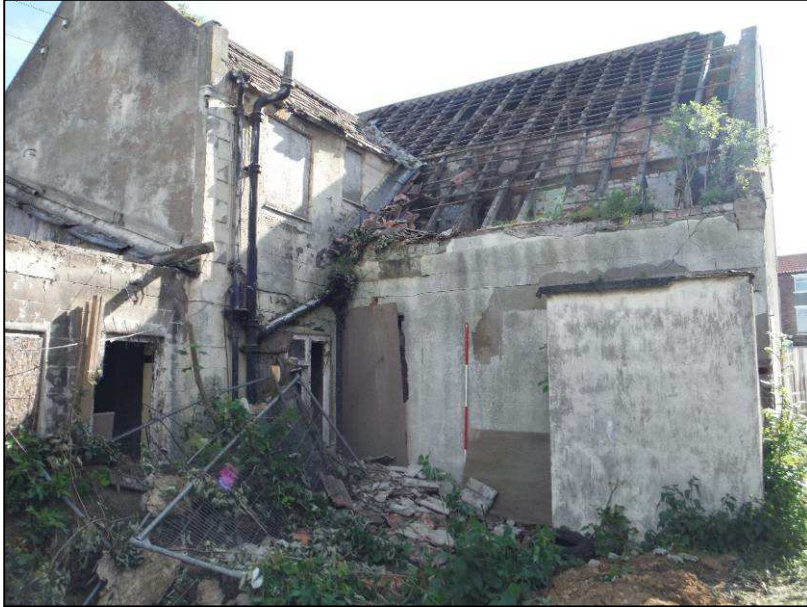
Plate 5 (Shot 12): Rear of building showing the lean-to extension, looking northeast (2m scale).
