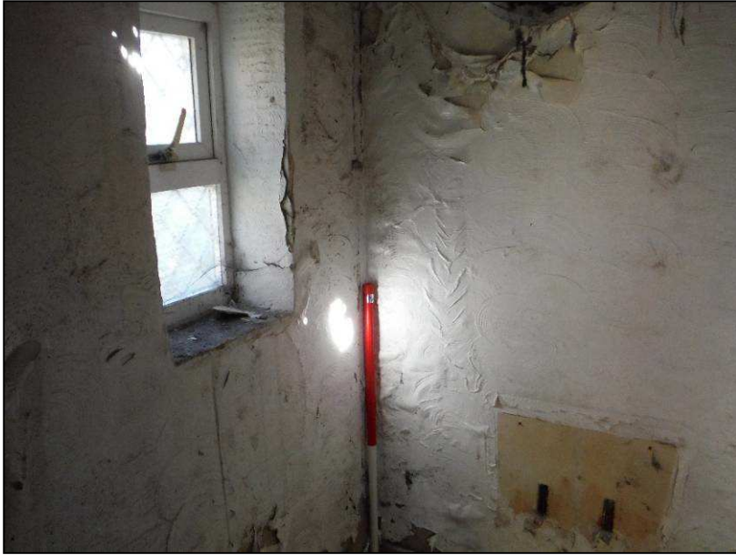
Plate 17 (Shot 45): Cut out of Room 3; probably a WC, looking northwest (1m scale)
