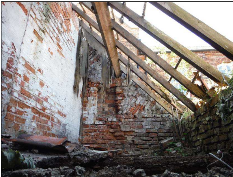
Plate 30 (Shot 77): Western extent of the lean-to showing blocked window and diagonal bond of the brickwork close to the roofline, looking south
