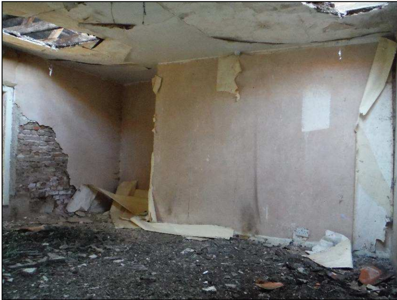
Plate 25 (Shot 70): Room 7, showing exposed brickwork on the southern elevation and the covered chimneystack on the western elevation, looking southeast
