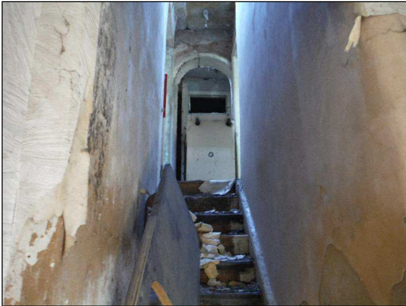
Plate 8 (Shot 65): Front entrance to the building showing staircase, looking west (2m scale)
