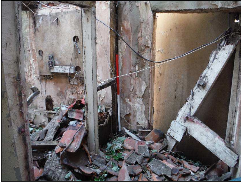
Plate 21 (Shot 74): Entrance to the extension from the rear of the property and the stud wall leading into the lean-to extension, looking west (1m scale)
