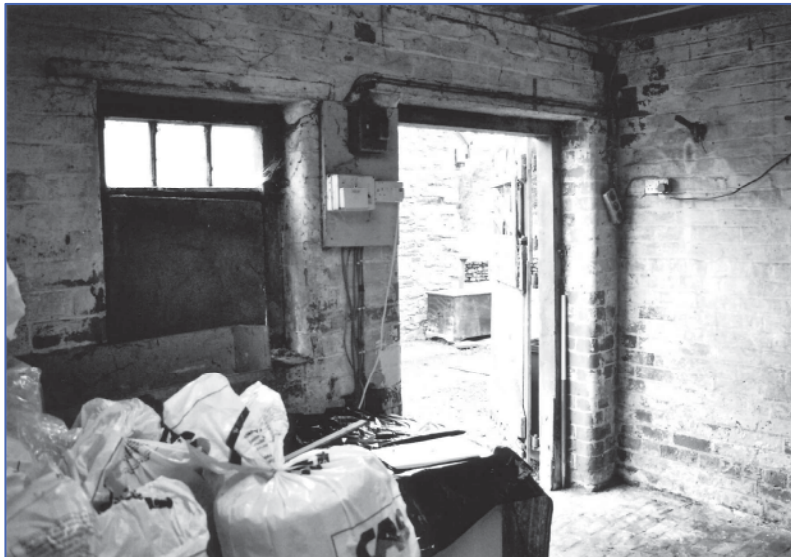
Plate 11: Interior view of the door and window in the lower storey of the east elevation, looking south
