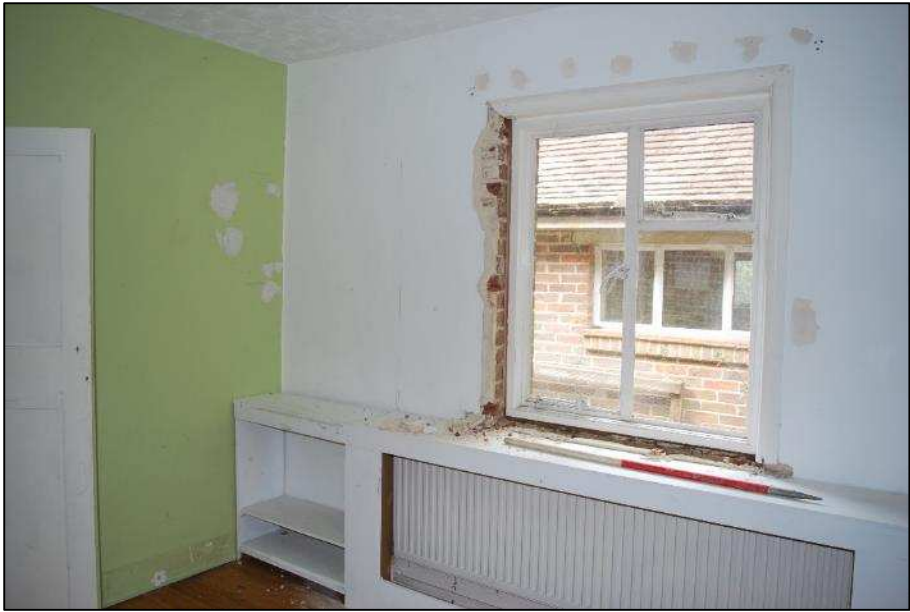
Plate 45 (Shot 387): Inbuilt storage in the bungalows dining room, looking west, 1m scale
