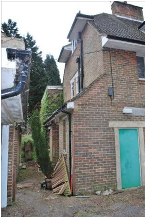
Plate 12 (Shot 32): Gap between Elevation E and the Garage and Bungalow, looking southeast 1m scale
