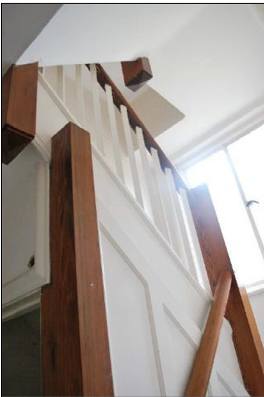
Plate 30 (Shot 209): Stairwell that provides access to the cellar, first and second floor, looking west
