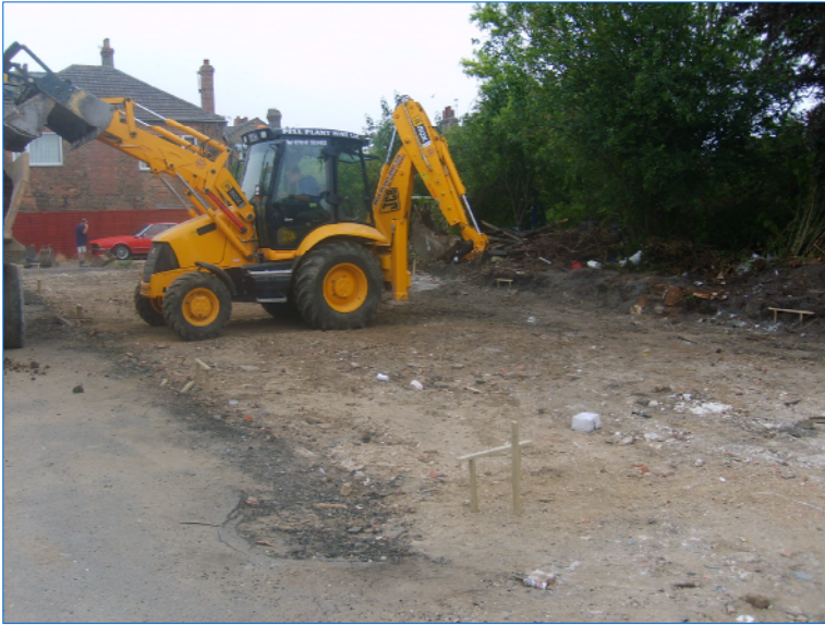
Plate 1: General view of the development area taken from junction between Ranters Row and track at southeast corner of site, looking northwest
