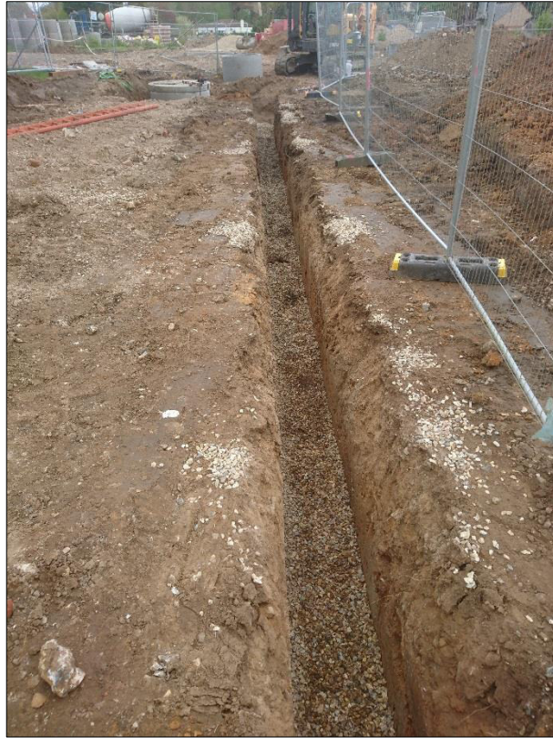
Plate 2: Example service run, looking south
