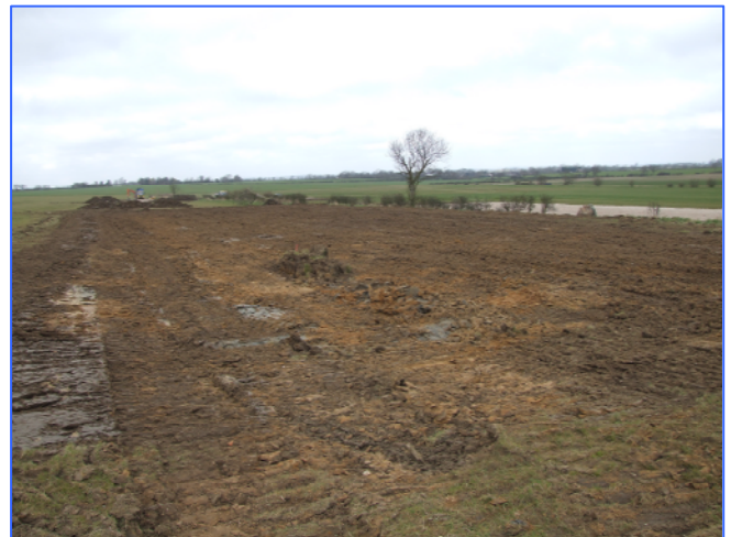
Plate 4: The stripped area of the south-eastern chicken shed, looking west. The south-western chicken shed is being machine stripped in the background, and the stoned up area of the north-eastern chicken shed is visible to the right of the shot.
