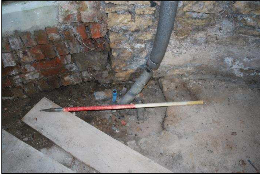
Plate 15 (Shot 66): Pipework coming through the floor and brickwork below inserted window, looking northwest (1m scale)
