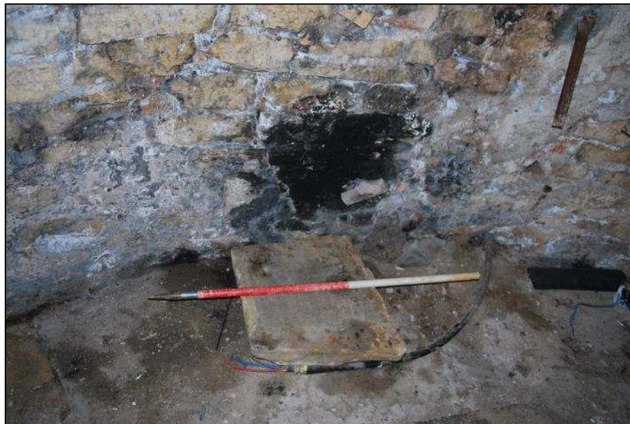
Plate 12 (Shot 67): Burnt area on ground floor, looking north (1m scale)
