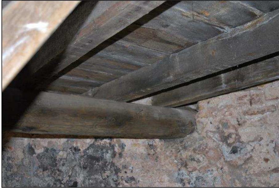
Plate 23 (Shot 44): Trunk used for a beam on the second floor, looking southeast
