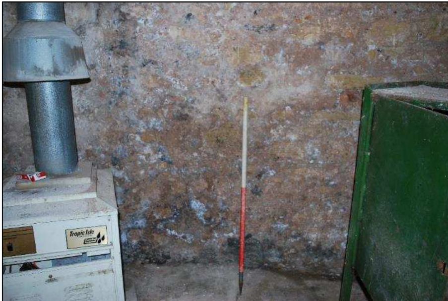
Plate 10 (Shot 75): Plasterwork falling away on the ground floor, looking southwest (1m scale)
