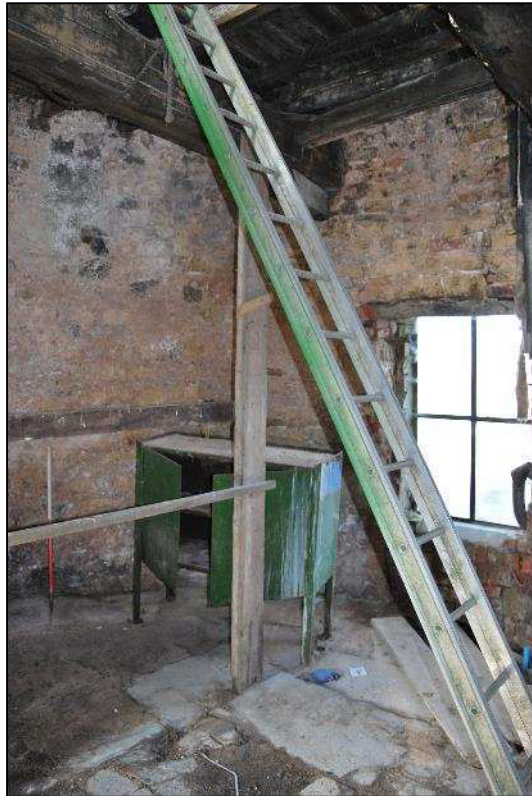
Plate 11 (Shot 70): General view of ground floor interior, showing patchwork of repairs to floor, looking east-southeast (1m scale)
