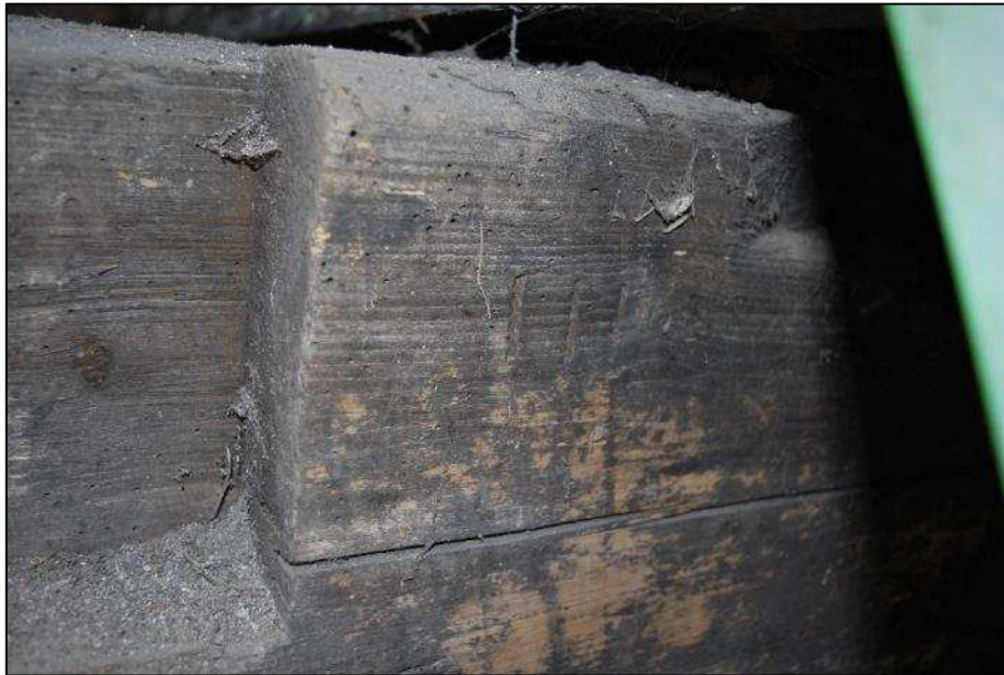
Plate 22 (Shot 59): Unused socket and assembly mark on the principal beam (looking southwest)
