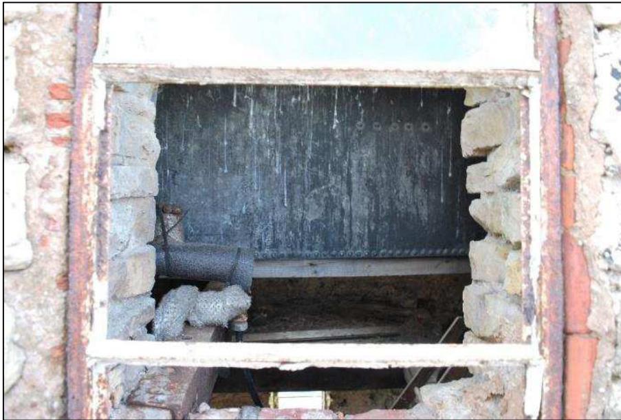
Plate 24 (Shot 9): Second floor of the building, viewed from the exterior, showing the inserted water tank and its supporting joists, looking southeast
