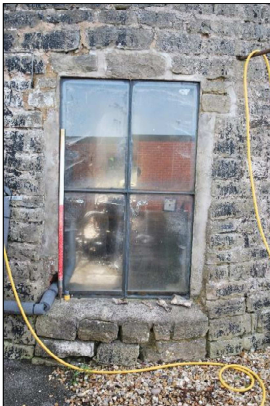
Plate 6 (Shot 21): Large four-light casement window inserted in place of a door, looking southeast (1m scale)
