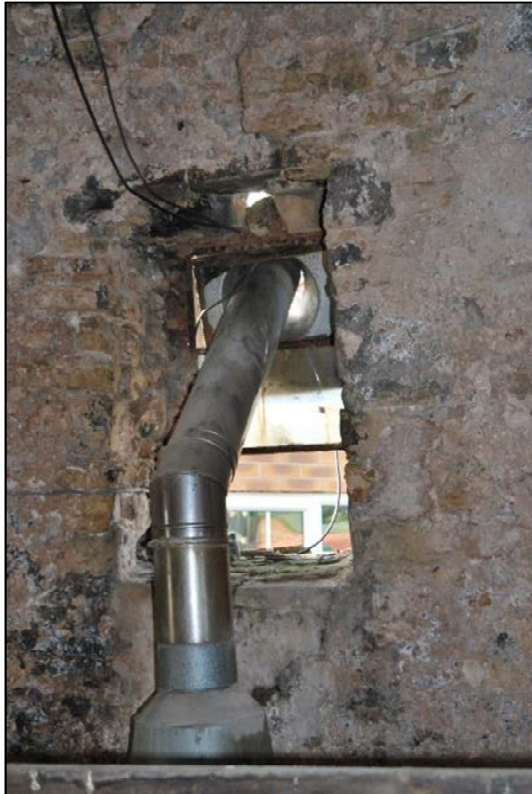
Plate 13 (Shot 69): Chimney from the boiler going through a ground floor window, looking southwest
