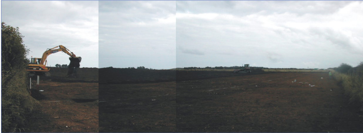
Plate 1: Well Site stripping underway. Photo taken from SW corner looking NE to E
