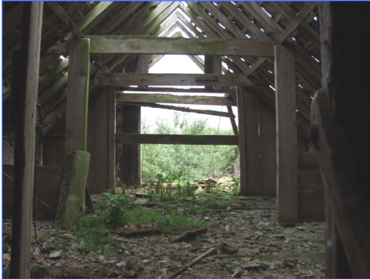
Plate 7: Hayloft above the stable block. Note the wooden partitions dividing the room into bays. Looking east-north-east.
