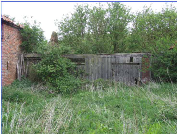
Plate 20: West elevation of the barn at the east end of the crew yard. Looking east-north-east.
