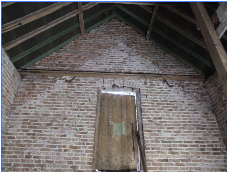
Plate 8: East internal elevation of the three storey threshing barn, showing the roof line of the adjacent stable/hayloft. Looking east-north-east.
