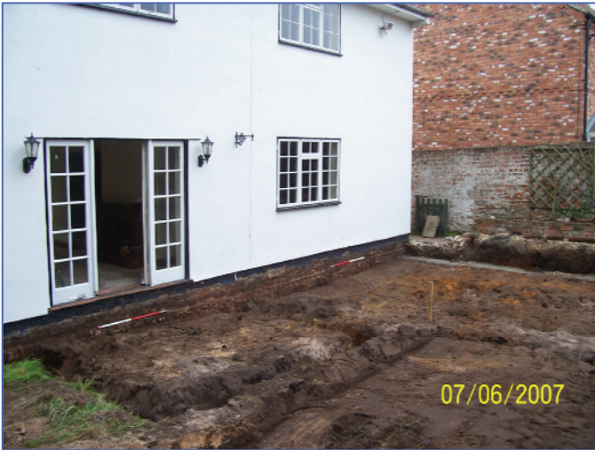
Plate 1: Foundation trenches excavated to the south of the existing farm house. Looking north-east
