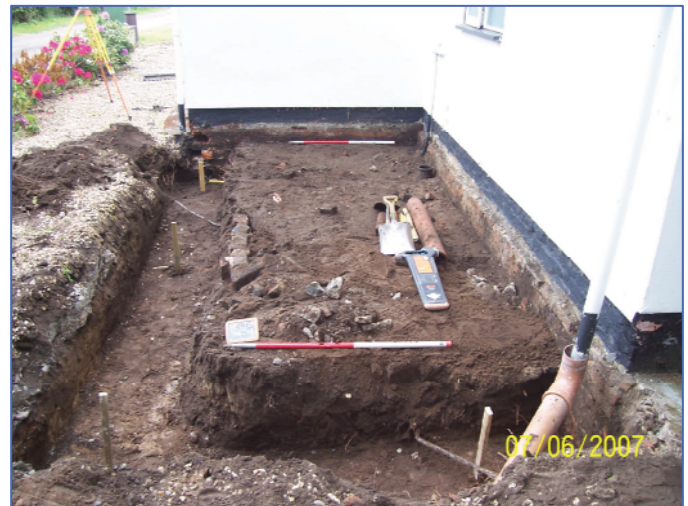
Plate 4: Foundation trenches excavated to the north of the existing farm house after removal of the brick boundary wall. Looking east-north-east.
