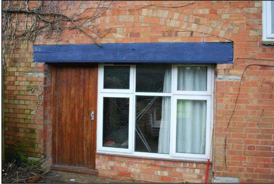
Plate 3 (Shot 60): Second doorway and window inserted into previous opening, looking northeast (1m scale)
