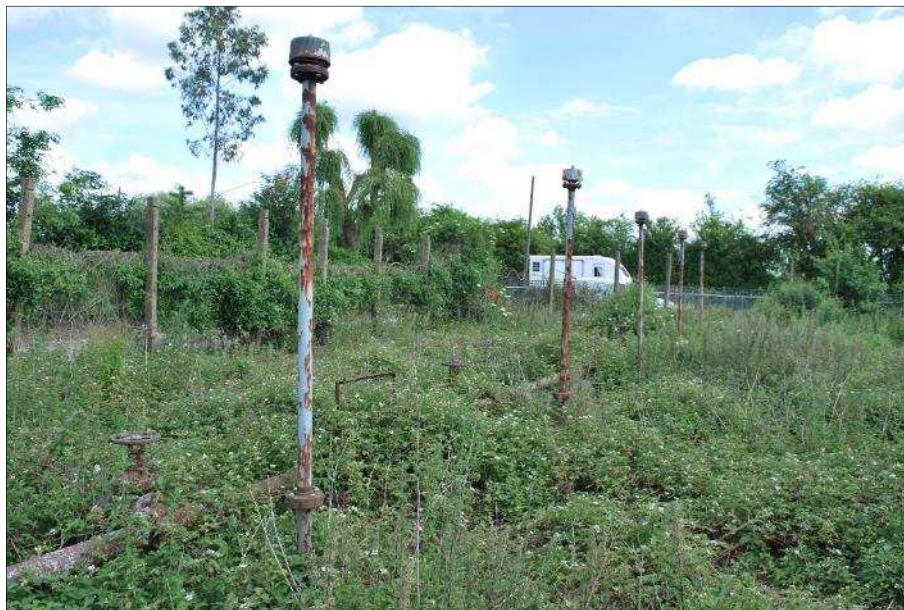
Plate 14 (Shot 41): Vertical above-ground vents and ground-level valves at north end of fuel tanks, looking northeast
