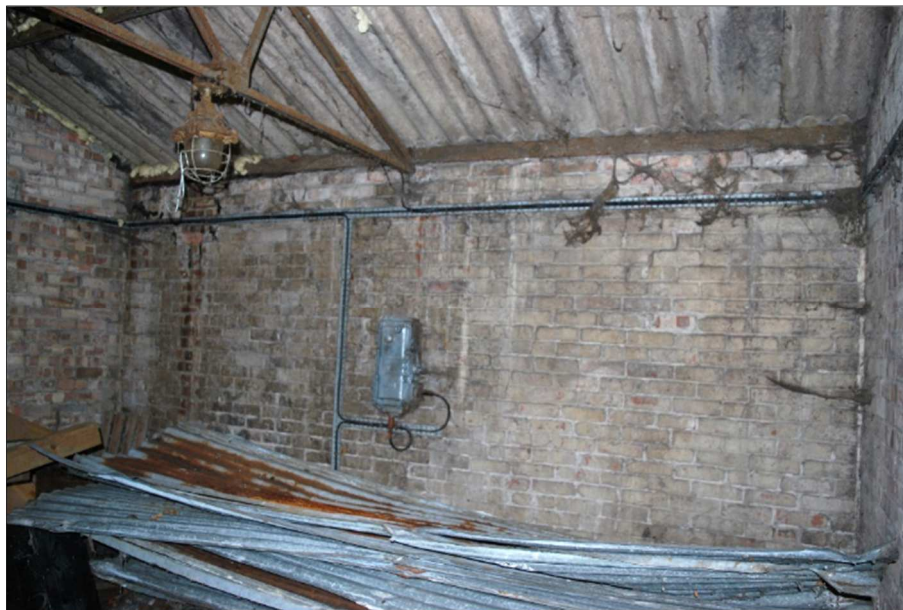
Plate 7: (Shot 23): General internal view showing corrugated metal stored within building, looking northwest
