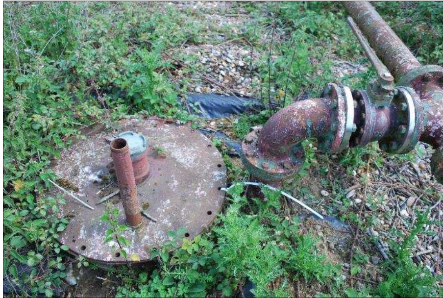
Plate 15: (Shot 37): Circular access vent and connecting pipework, looking east
