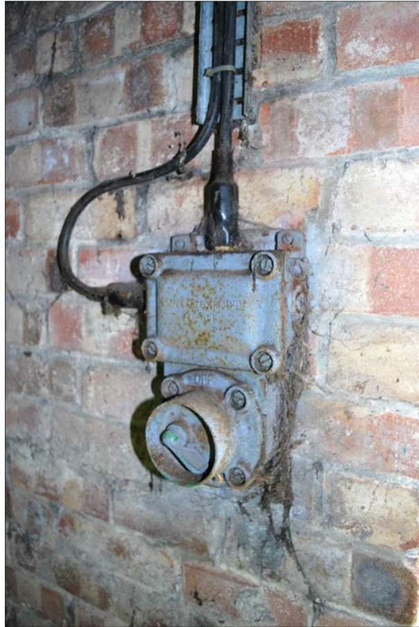
Plate 10 (Shot 14): Metal electrical switch panel on eastern wall, looking northeast
