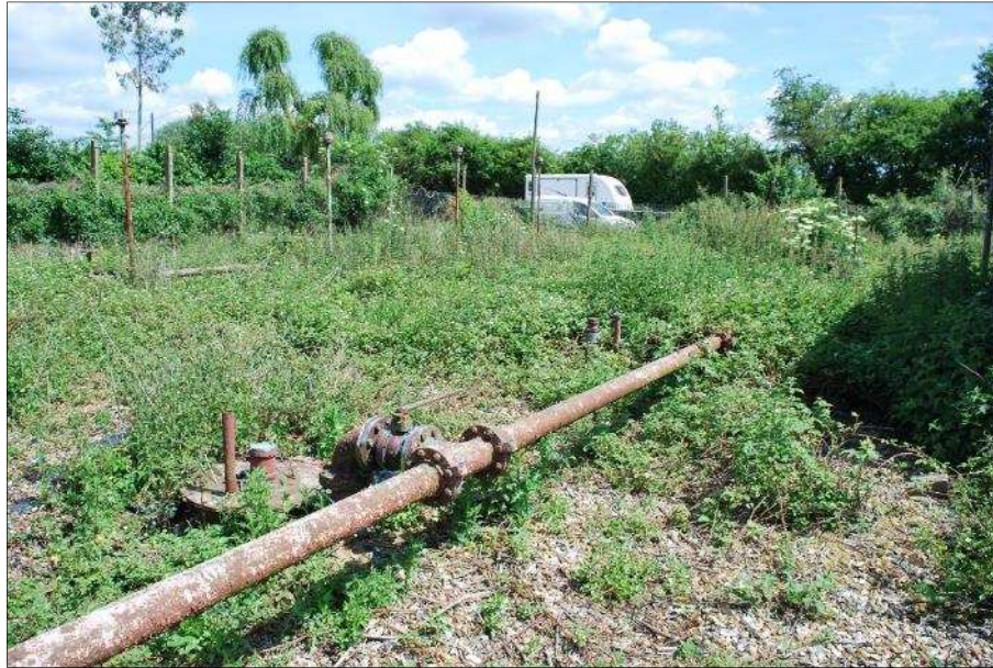
Plate 13 (Shot 35): Network of above-ground pipes associated with fuel tanks, looking northeast
