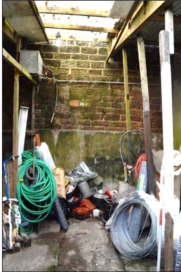
Plate 18 (Shot 95): Interior view of lean-to Building 3, showing stone wall of barn (Building 1) and manuring gully, looking west (1m scale)
