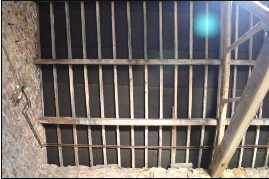
Plate 24 (Shot 48): General view of roof structure at northeast corner of barn (Building 1, Room 1a), looking east
