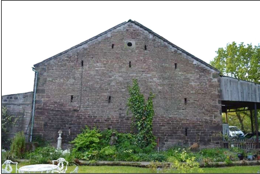
Plate 7 (Shot 29): North elevation of barn (Building 1), showing owl hole, breather slits and eaves (1m scale)
