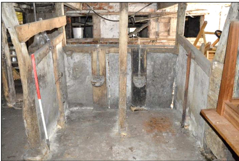
Plate 41 (Shot 67): Interior of Room 1b, wood and stone flag animal stalls with tethering posts and rings and drinkers, looking east (1m scale)
