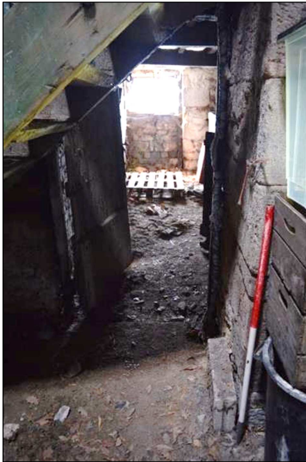
Plate 37 (Shot 58): General view of ground floor feeding passage from Room 1a to animal accommodation at southwest of building (Room 1b), looking south towards blocked door in south gable end of barn (1m scale)
