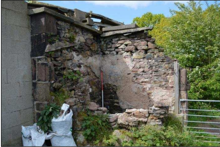
Plate 71 (Shot 111): East part of Building 8, possible former toilet, showing residual plaster and eaves scar of former pitched roof, looking west (1m scale)
