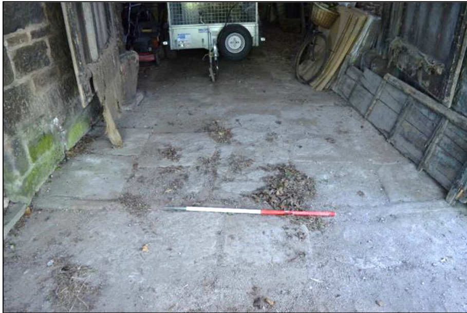
Plate 19 (Shot 44): Detail of flagstone flooring at west entrance to barn (Building 1), looking east (1m scale)
