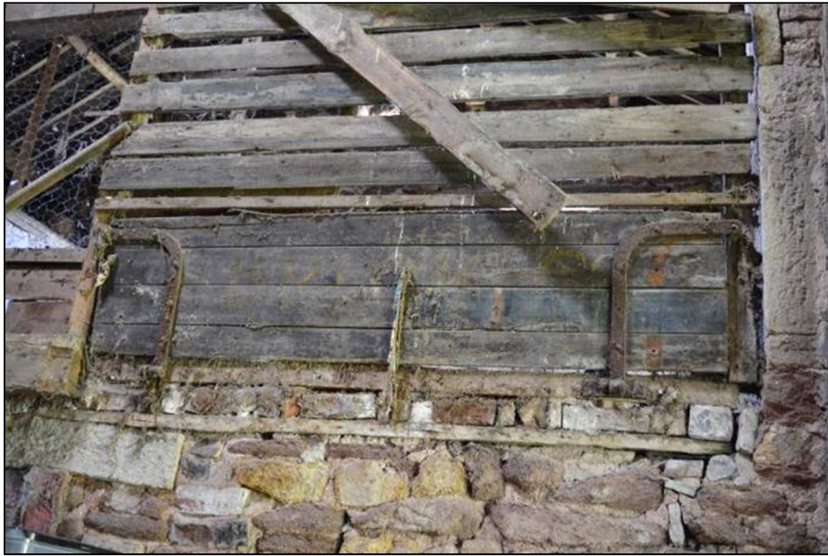
Plate 36 (Shot 57): Barn (Building 1, Room 1a) interior detail, showing stonework of southern partitioned area and drop down hatch, looking south
