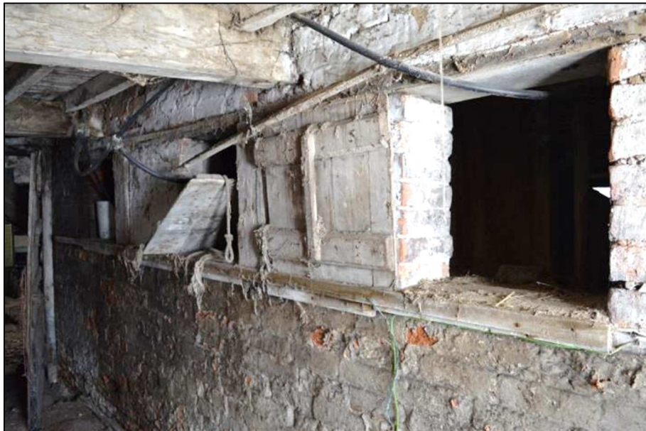
Plate 34 (Shot 61): Interior of ground floor southwest corner of barn, detail of brick wall between Rooms 1b and 1c with adjustable openings, looking northeast
