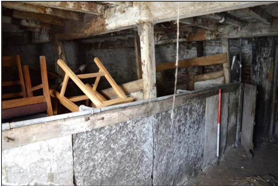
Plate 39 (Shot 59): Interior of ground floor animal accommodation in Room 1b, showing stone and wood stalls, looking northwest (1m scale)
