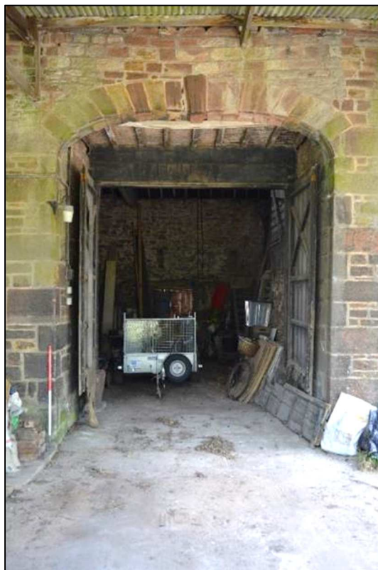
Plate 10 (Shot 35): Detail of west elevation of barn (Building 1), arched opening over double doors, looking east (1m scale)
