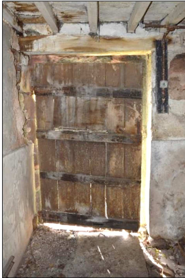
Plate 47 (Shot 131): Interior of ground floor Room 1c, animal accommodation, east doorway of south gable end of barn, looking south
