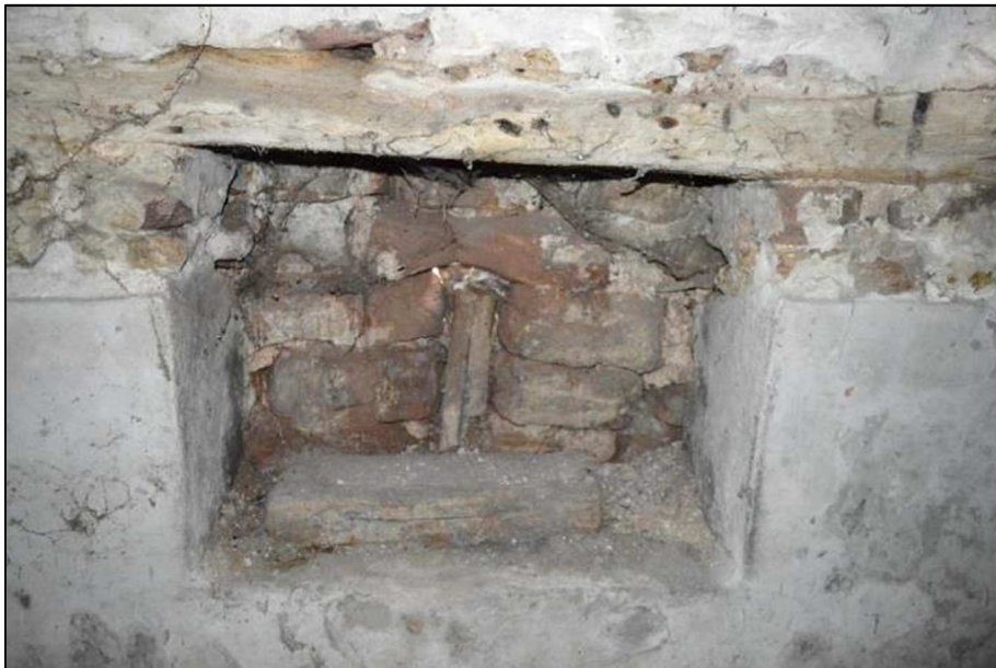
Plate 45 (Shot 66): Detail of Room 1b, low recess in west wall of barn and blocked breather slit, looking west
