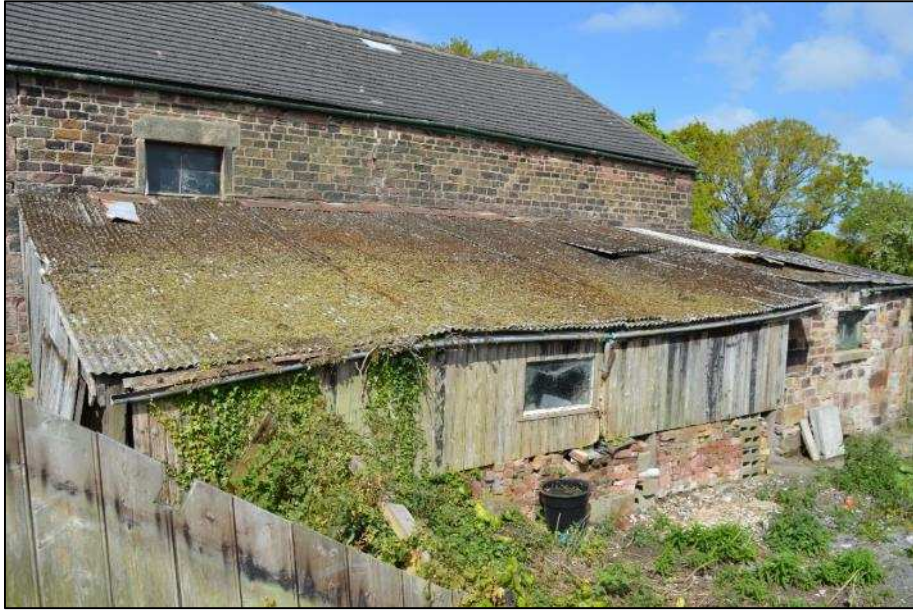
Plate 14 (Shot 100): East elevation of barn (Building 1) and adjoining lean-to Buildings 3 and 4, looking northwest
