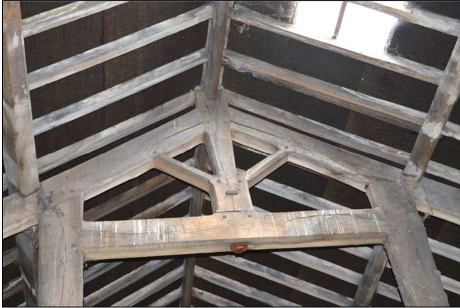
Plate 30 (Shot 81): Interior of barn showing detail of roof truss to north of paired barn doors, looking north
