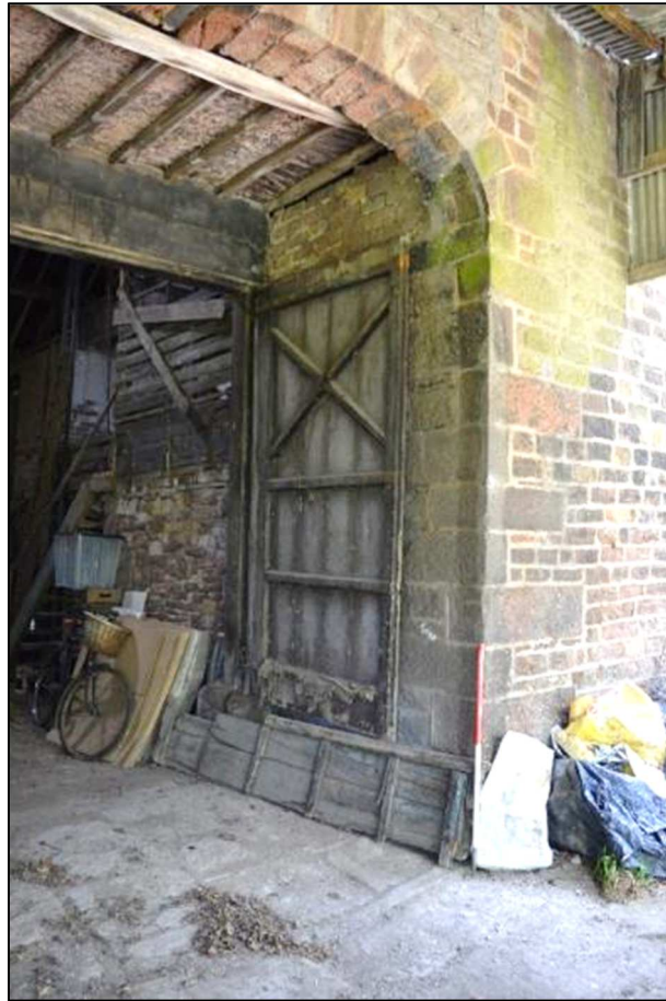
Plate 12 (Shot 38): Detail of entrance at west side of barn (Building 1), including wooden threshold and carved stone to accept it, looking southeast (1m scale)
