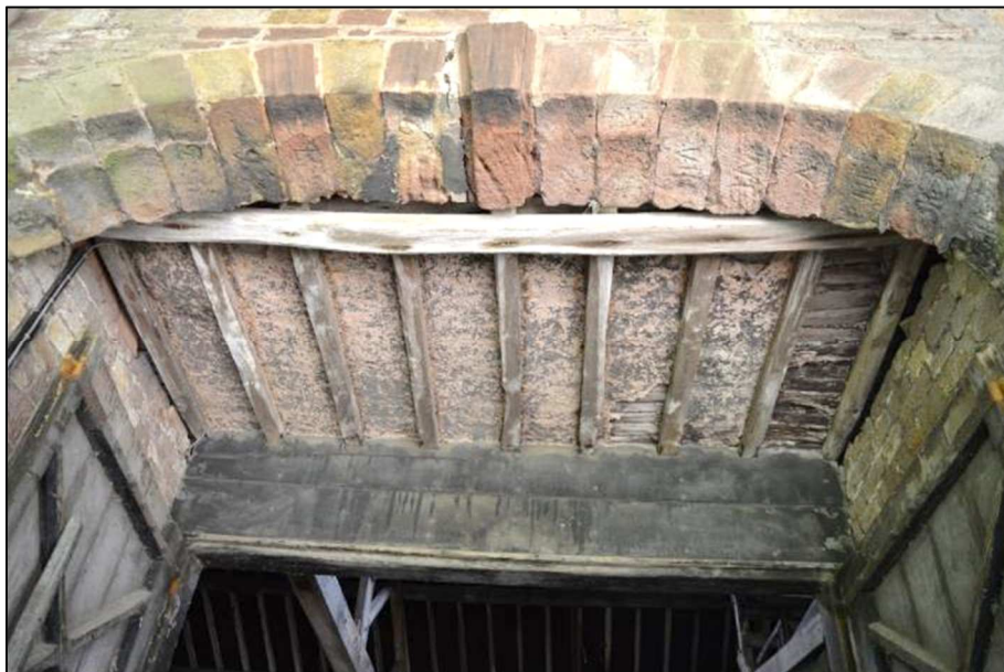
Plate 13 (Shot 43): Detail of porch over entrance at west side of barn (Building 1), including carved numbers and numerals on arch relating to its construction, and lath and plaster ceiling, looking east
