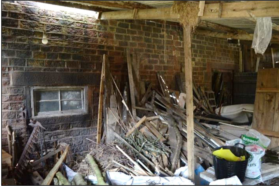
Plate 16 (Shot 92): Interior of lean-to Building 4 showing window and door of east wall of barn (Building 1), looking northwest (1m scale)
