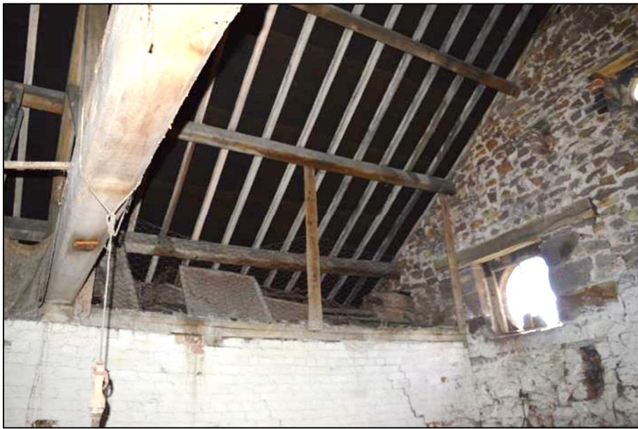
Plate 25 (Shot 73): Interior of barn, detail of brick partition wall and roof structure, looking southeast
