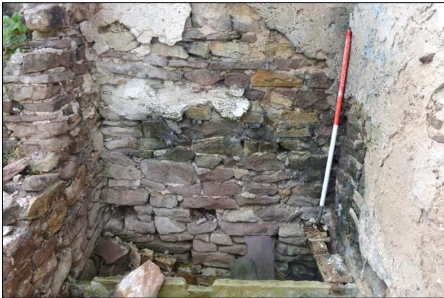
Plate 72 (Shot 109): Interior of east part of Building 8 showing stone structure with partially extant timbers, possibly former toilet, looking south (1m scale)
