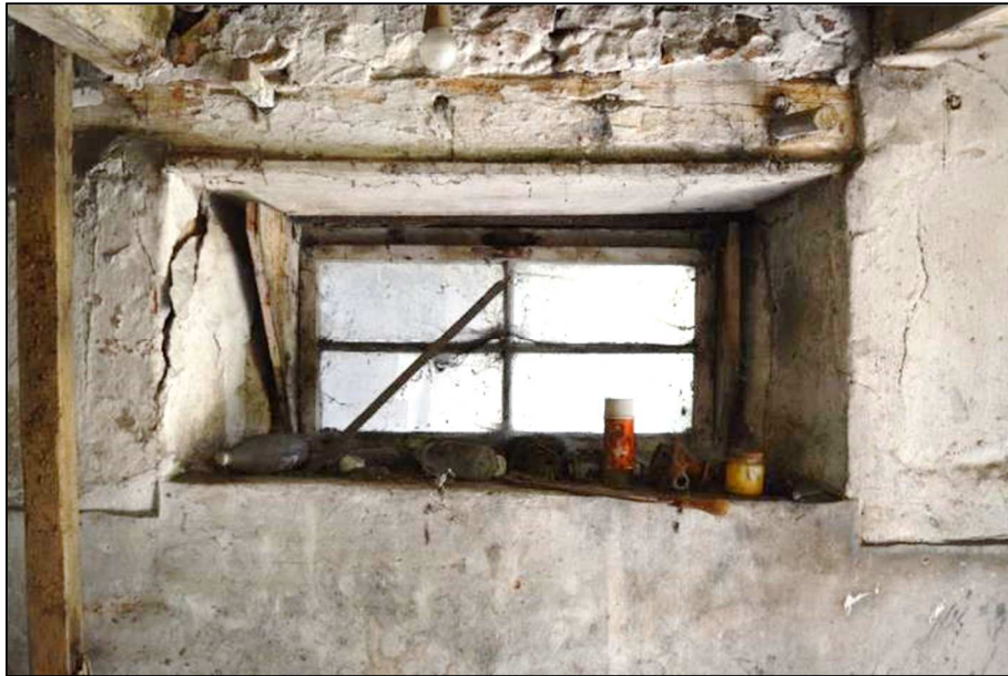
Plate 51 (Shot 129): Interior ground floor of Room 1c, detail showing recessed window forming shelf and possible tack or equipment pegs over, looking east
