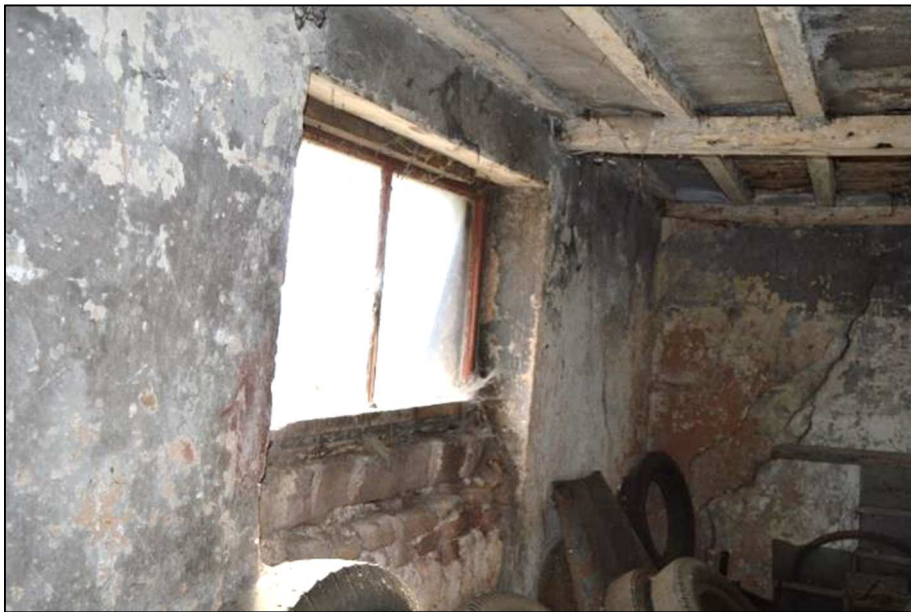
Plate 56 (Shot 84): Interior of barn first floor Room 1e showing possibly partly blocked pitching hole or door in east wall, looking southeast
