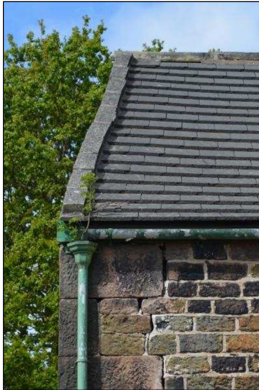
Plate 9 (Shot 106): Detail of roof and guttering of barn (Building 1) at southeast corner, looking west
