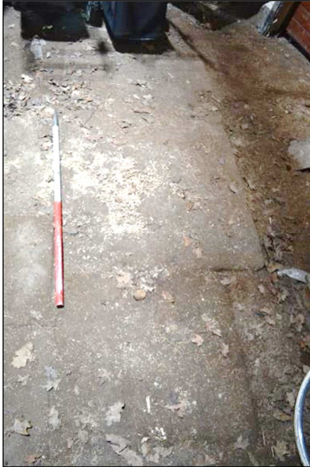
Plate 23 (Shot 50): Mixed concrete, brick and earth flooring between opposing doors of barn (Building 1, Room 1a), looking west (1m scale)
