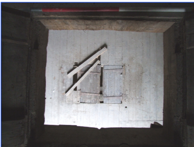
Plate 15: View through hatch on second floor, showing the hatch on the first floor below.
