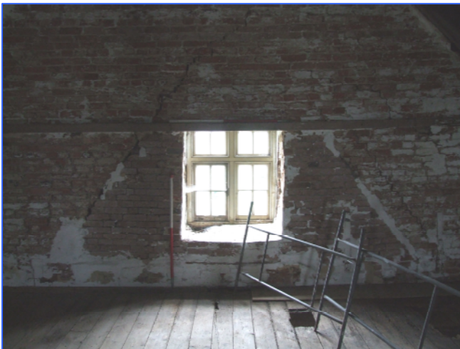
Plate 14: Window at the south end of the second floor, showing the cracks evidencing the subsidence of the south wall. Looking south.
