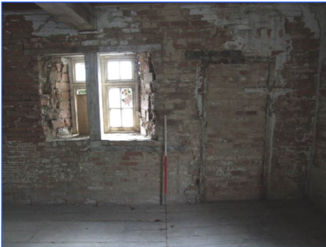
Plate 11: South wall of the first floor, showing the window and blocked doorway, looking south.
