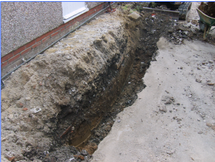
Plate 3: Working shot during excavation of footings to the east of the existing building. Looking south-east.
