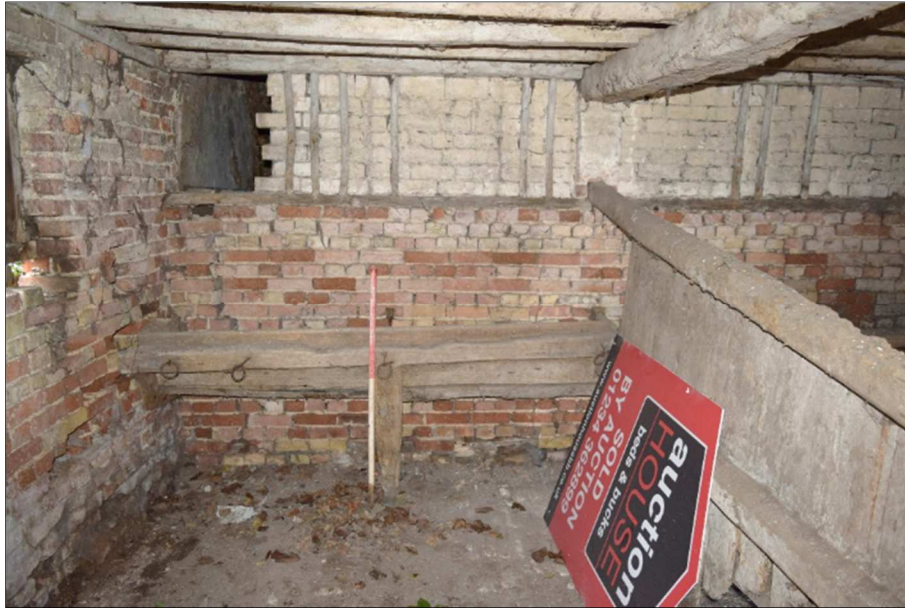
Plate 13 (shot 16): Representative view of the southwest stall showing wooden partition above the bricks. Looking northwest, 1m scale
