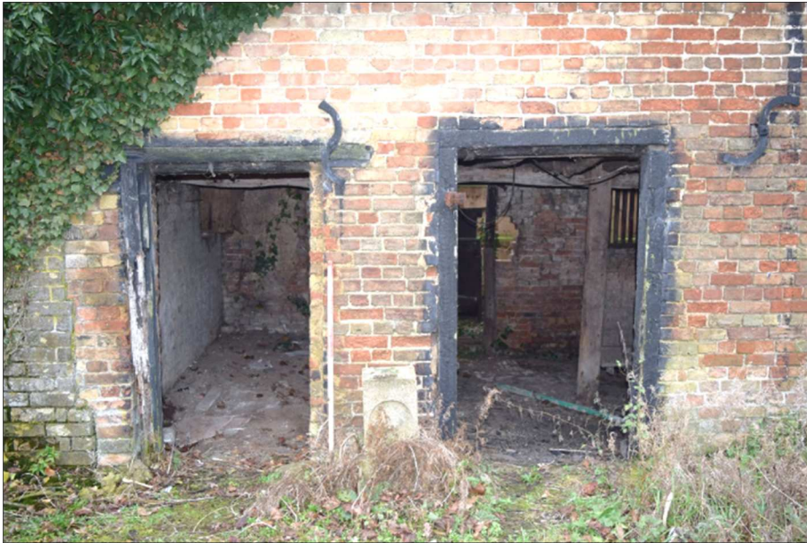
Plate 5 (shot 11): Openings on northeast elevation also showing abutting barn to the left. Looking south, 1m scale
