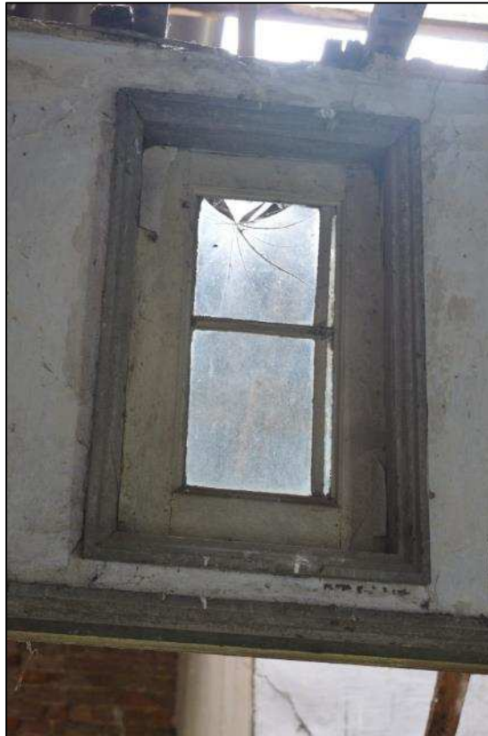
Plate 26: (Shot 186) Light above internal door to first floor Room 8 of Farmhouse A, looking south towards landing and stairs
