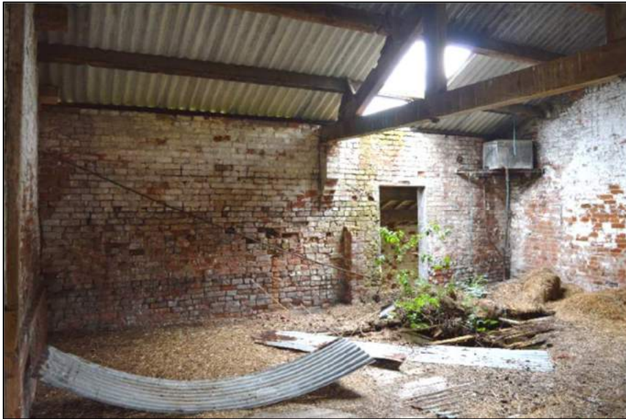
Plate 47: (Shot 196) First floor Room 14 of Barn B showing doorway to Building C, looking southwest
