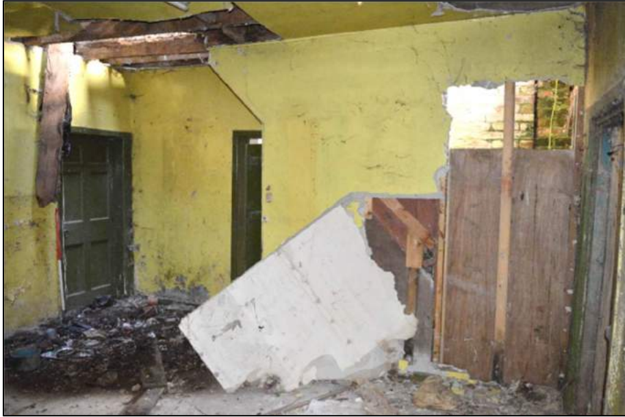
Plate 16: (Shot 156) Interior of Room 3, looking northeast towards stairs 11 and doors to Room 1 and 4 (1m scale)
