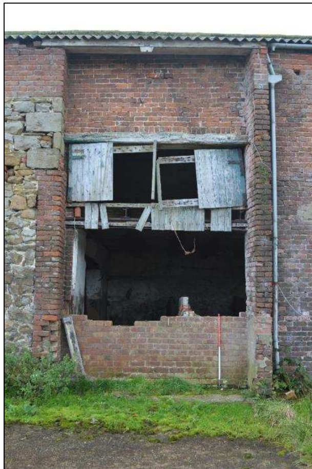
Plate 34: (Shot 22) Partially-blocked opening in north elevation of Barn B, wooden shutters to first floor and eaves scar, looking south (scale 1m)
