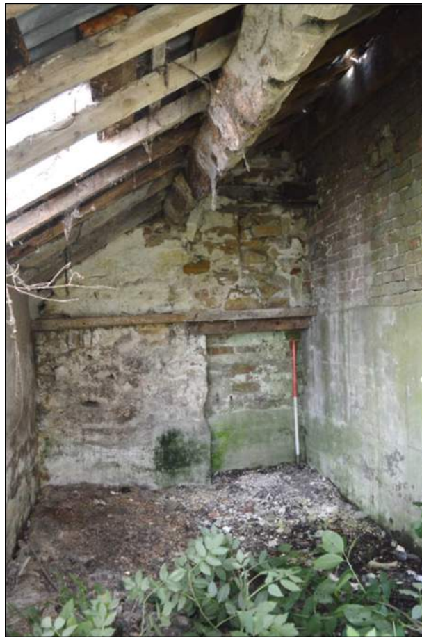
Plate 65: (Shot 64) Interior of Building D, showing re-used roof timber and blocked openings in west gable end, looking west (1m scale)
