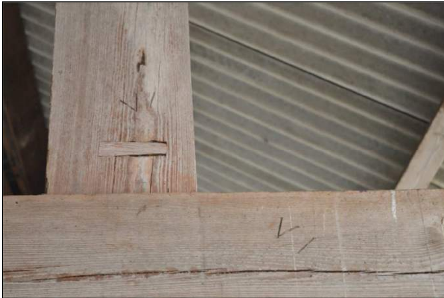
Plate 56: (Shot 206) Detail of truss construction and carpenter's marks in Room 15, looking east
