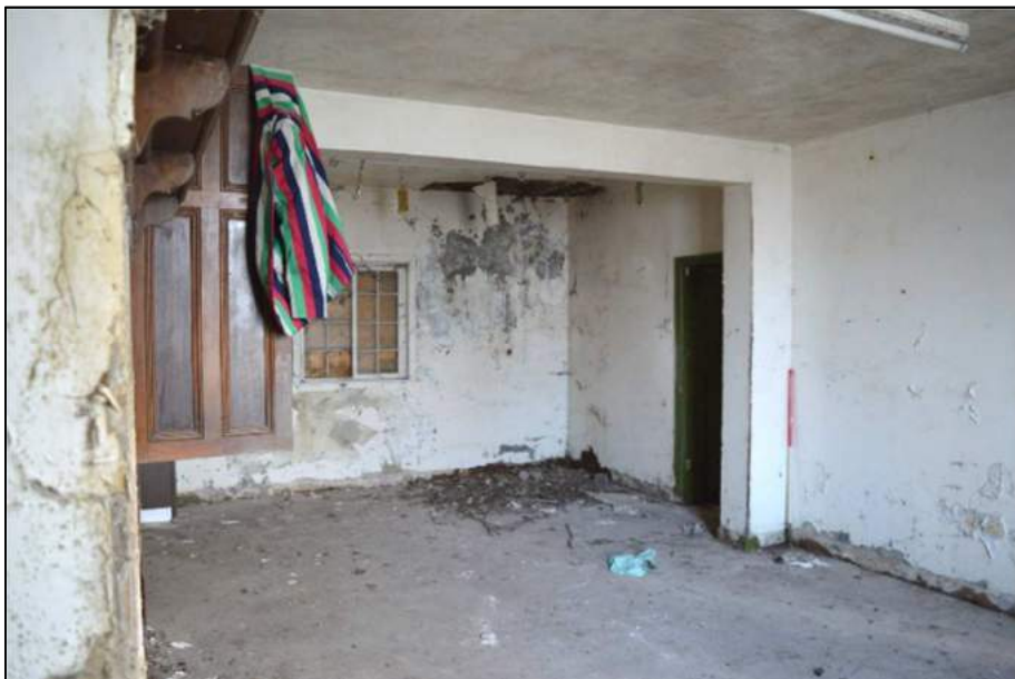
Plate 13: (Shot 145) General view of Room 4 of Farmhouse A, looking southeast, showing door to Room 3 (1m scale)
