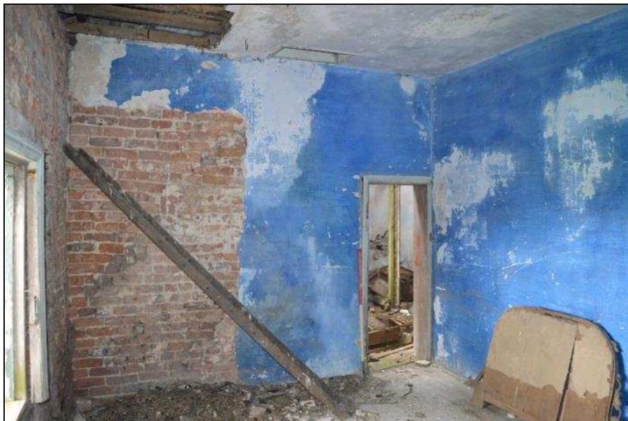
Plate 20: (Shot 169) First floor Room 13, Farmhouse A, looking west towards stairs and landing (1m scale)
