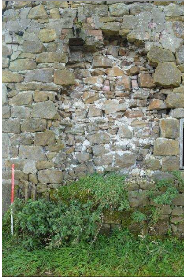
Plate 37: (Shot 36) Deterioration of facing stonework of north elevation of Barn B, looking south (1m scale)
