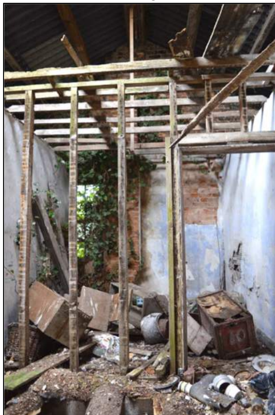
Plate 27: (Shot 179) View west from landing through partition wall and doorway to Room 9 in first floor of Farmhouse A
