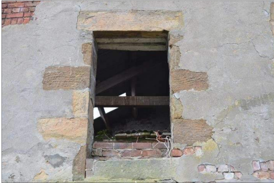
Plate 40 (Shot 42) First floor opening in east gable of Barn B, looking west
