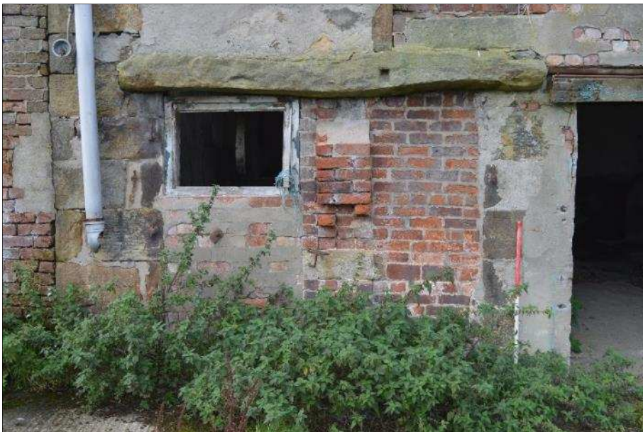
Plate 39: (Shot 43) Detail of east gable of Barn B, showing re-used stone lintel over blocked and partially-blocked doors and stone quoins at southeast corner of barn, looking west (1m scale)
