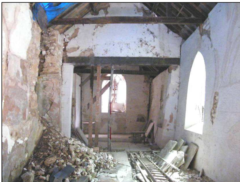
Plate 9 (shot 24): General view of the interior, looking east towards the chancel, 2m scale
