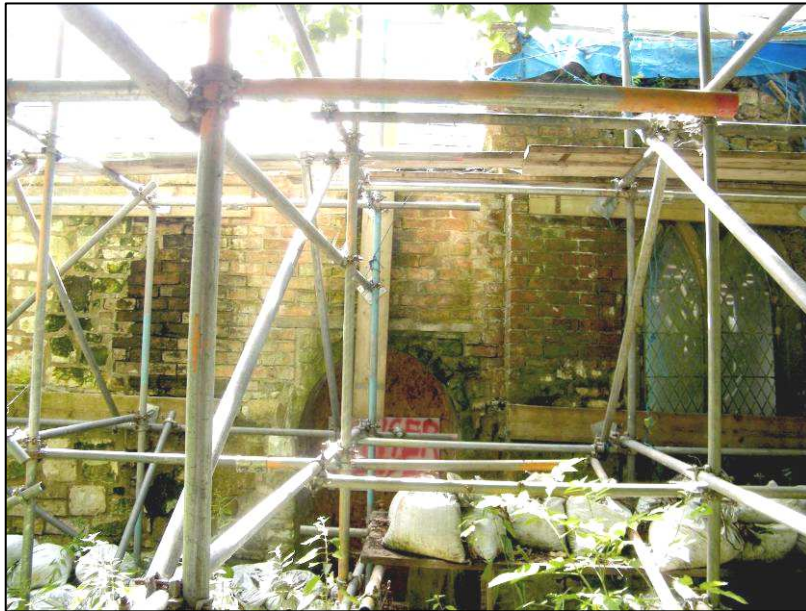
Plate 8 (shot 43): North elevation showing repair work in brick and boarded up doorway
