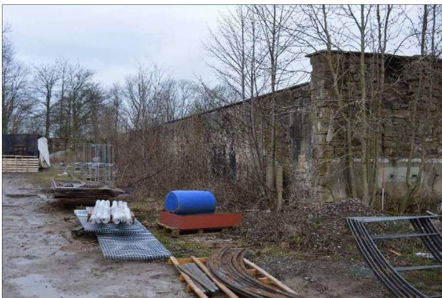
Plate 85 (shot 140): South partition of the weaving shed. The yard was once occupied by the former spinning and carding room. Looking west, 1m scale
