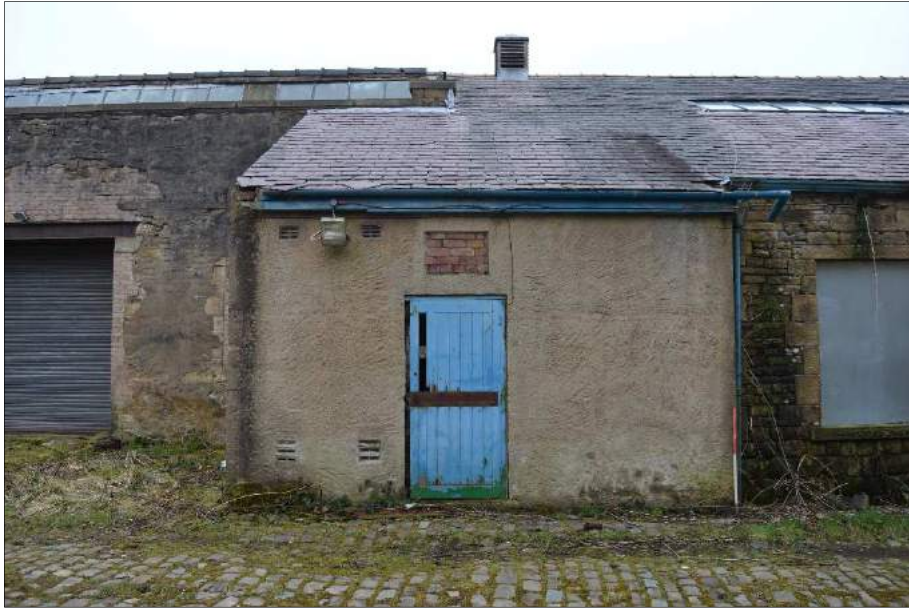
Plate 56 (shot 51): Small extension between the engine house and the former weft warehouse. Looking southeast, 1m scale
