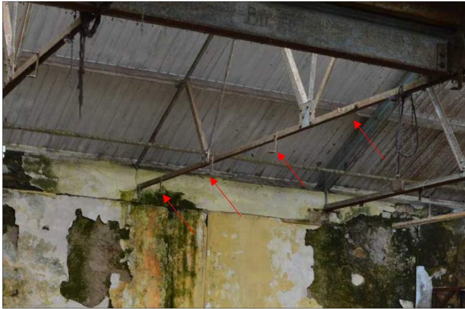
Plate 24 (257): Metal L-shaped brackets attached to the horizontal truss beam (see arrows). Looking south
