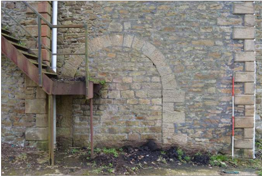
Plate 3 (shot 377): Blocked arched opening to former walk on the northwest elevation. Looking southeast, 2m scale
