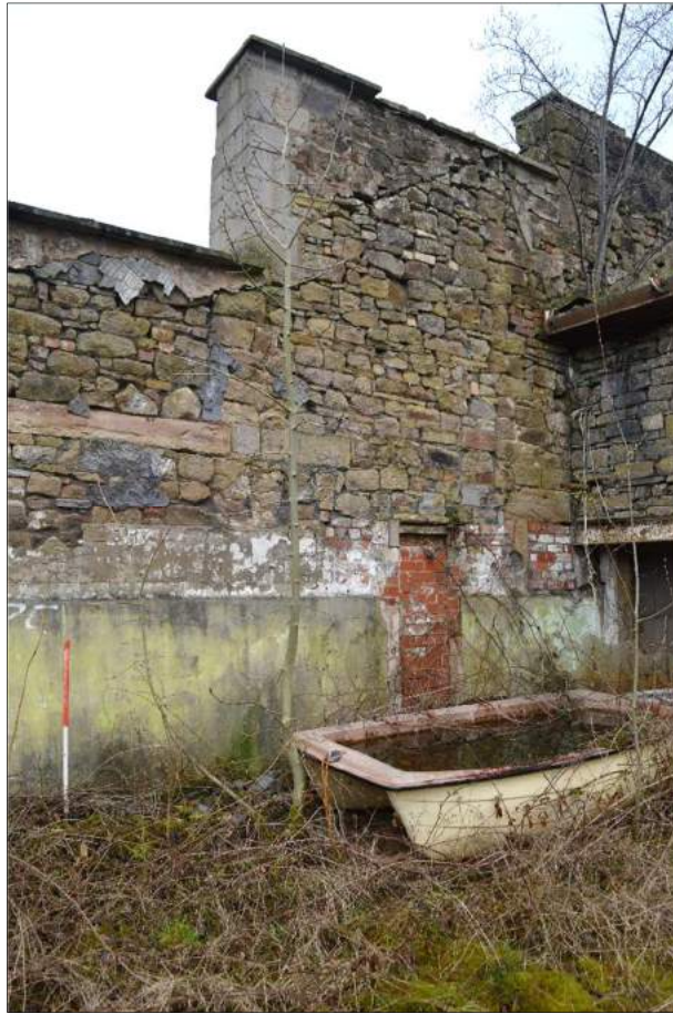
Plate 84 (shot 137): North elevation showing roof scar of demolished mill. Looking northwest, 1m scale
