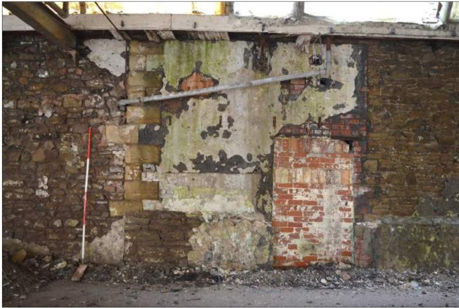
Plate 80 (shot 156): Quoins and plinth of original spinning mill and blocked access between the former spinning department and the carding room. Looking northwest, 2m scale
