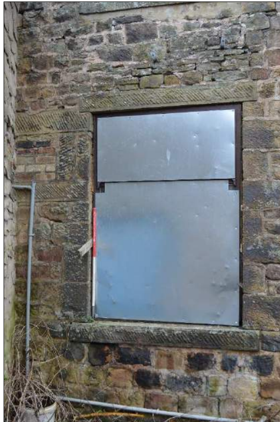
Plate 34 (shot 28): Blocked potential bearing box left of the window. Looking north, 1m scale
