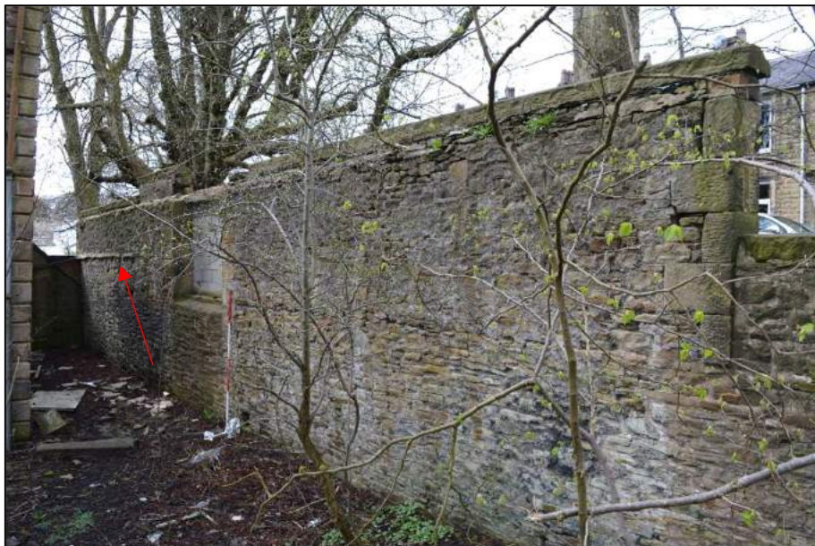
Plate 7 (shot 394): Boundary wall and former north elevation of 1910 structure. Arrow points to remains of roof structure of demolished lean-to. Looking northwest, 2m scale
