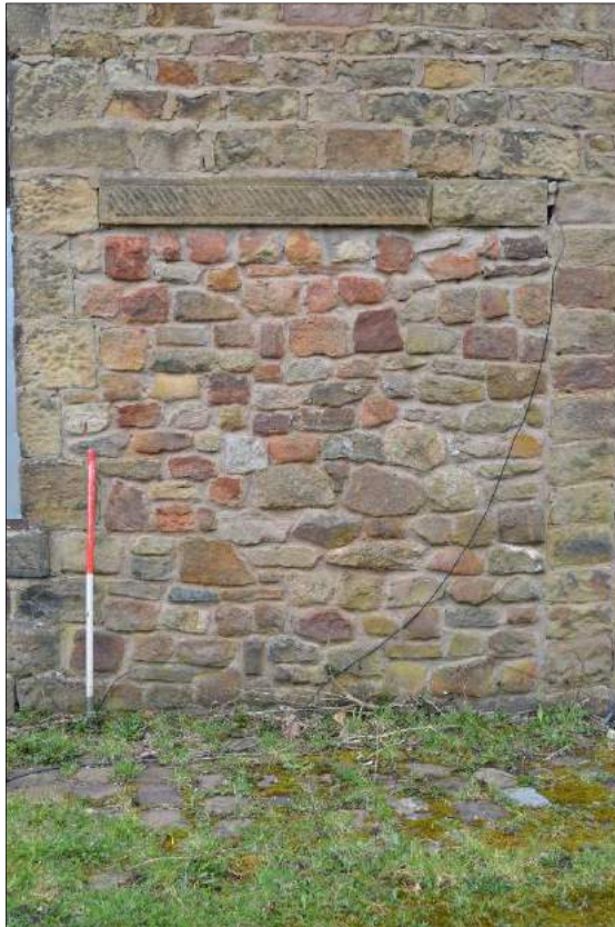
Plate 35 (shot 15): Blocked up later opening on ground floor. Looking north, 1m scale
