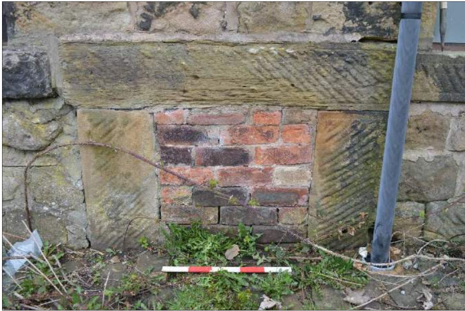
Plate 33 (shot 20): Blocked up opening for potential bearing box or flue. Looking north
