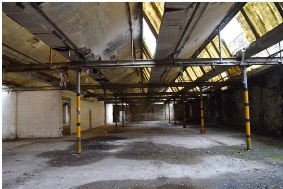
Plate 79 (150): Former carding room north of the later breeze block partition. Looking northeast, 2m scale
