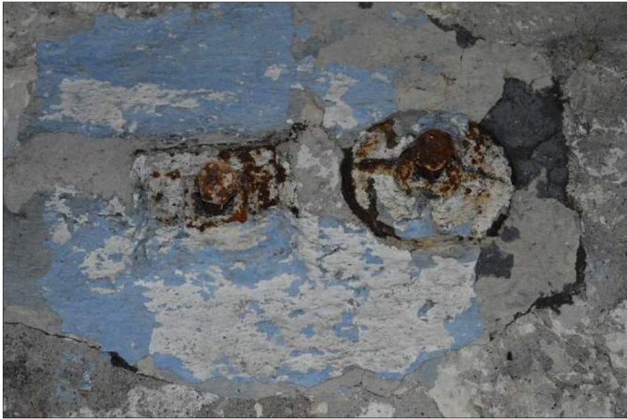
Plate 22 (shot 291): Small patress plates potentially related to a hoist on the south elevation. Looking southeast
