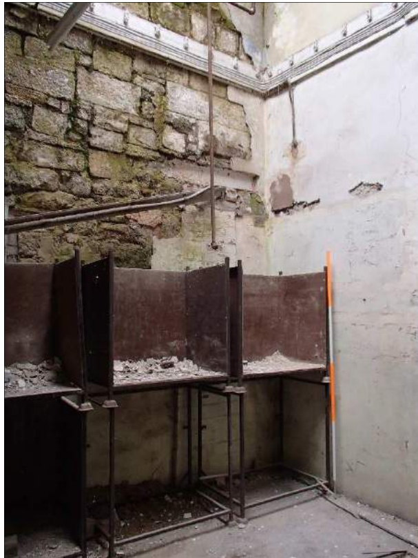
Plate 55 (shot 434): Bricked up tall opening in the corner behind the metal booth. Looking northwest, 2m scale
