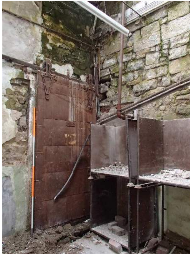
Plate 54 (shot 435): Early fire door from the mill days in the hoist and staircase. Looking south, 2m scale
