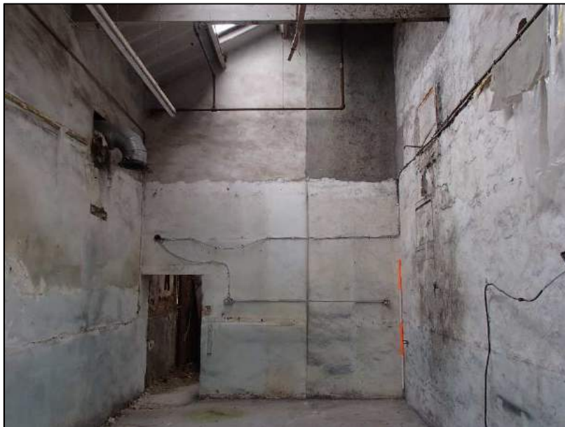
Plate 53 (shot 430): Bearing boxes on the south and north partition wall. Looking west, 2m scale
