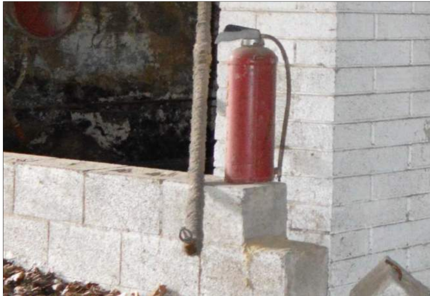
Plate 14 (shot 296): Part of sprinkler system showing intact sprinkler bulb and pipe with potential asbestos lagging.
