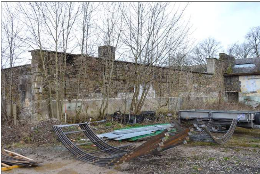
Plate 83 (shot 139): North elevation and partition wall to former mill. Looking northwest, 1m scale
