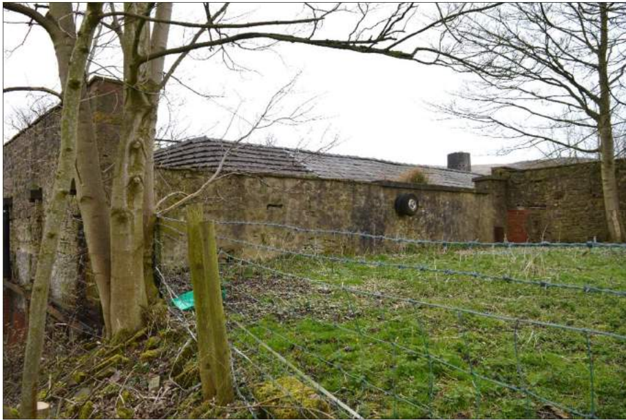
Plate 86 (shot 185): South elevation of the weaving shed and west elevation of former spinning and carding room to the left. Looking north
