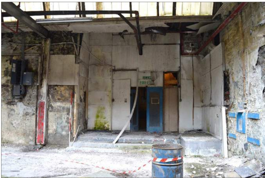
Plate 65 (shot 208): Southeast partition wall into the former spinning/weaving department. Looking northwest, 2m scale
