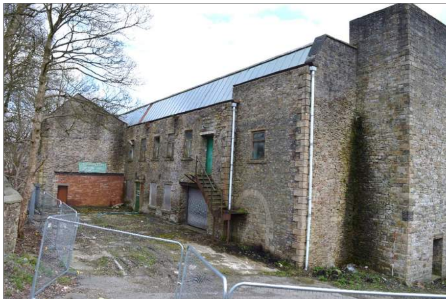
Plate 1 (shot 375): General view of Building A with later extension to the left. Looking southeast, 2m scale
