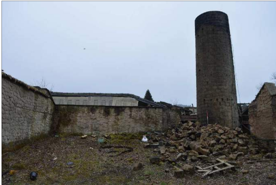
Plate 94 (shot 40): General view of the partly demolished chimney, remains of a flue situated below the scale, hidden by debris. Looking southeast, 1m scale
