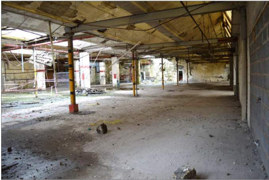
Plate 88 (shot 171): Steel column structure with steel girders and roof trusses. Looking northeast
