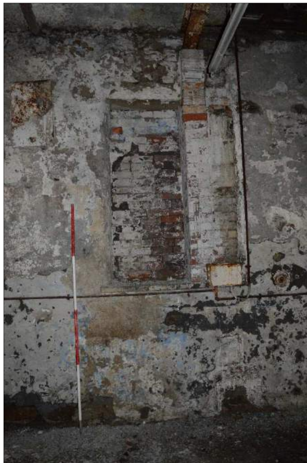
Plate 21 (shot 295): Blocked window of the earliest mill with later pilaster support for the RSJ above. Looking southeast, 2m scale
