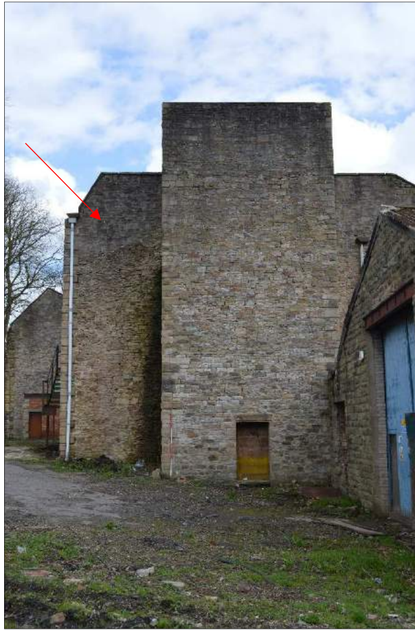
Plate 11 (shot 373): Southwest elevation revealing later repair work on the mill and showing the later ventilation shaft. Looking northeast, 2m scale
