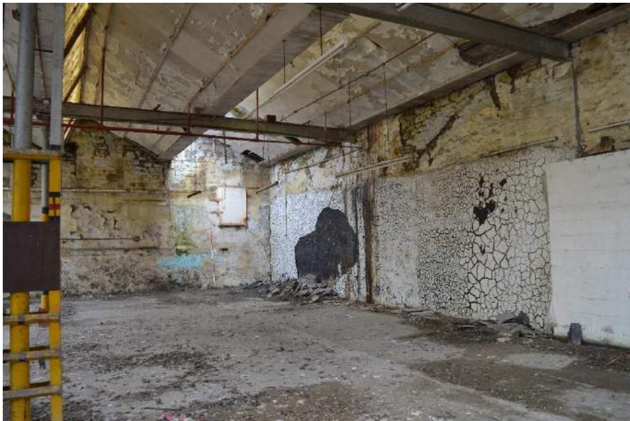
Plate 91 (shot 203): Southeast corner showing faint roof scars on the south partition wall. Looking east, 2m scale
