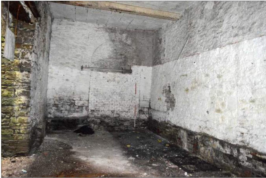
Plate 18 (shot 330): The full height of the arched opening on the mill's north elevation. Looking north, 2m scale
