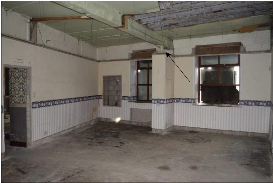
Plate 39 (shot 117): Cast-iron column hidden behind breeze blocks as shown by the arrow. Also notice the original floor joists seen in the ceiling. Looking southeast, 1m scale
