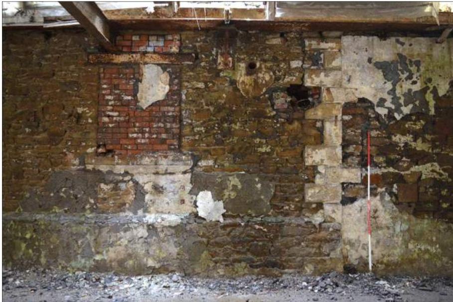
Plate 81 (shot 157): Bricked up earlier opening, plinth and quoins of original mill. Looking northwest, 2m scale
