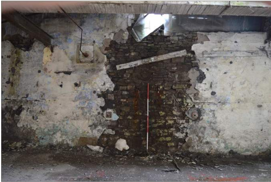
Plate 82 (shot 159): Former bearing box on the north wall. Looking northwest, 2m scale
