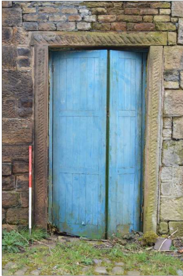
Plate 58 (shot 49): Close up of original door with dressed stone surround with cable moulding. Looking southeast, 1m scale
