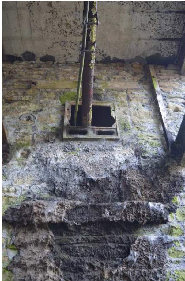
Plate 10 (shot 400): Iron bearing box within an earlier blocked up opening on the south elevation. Looking northwest
