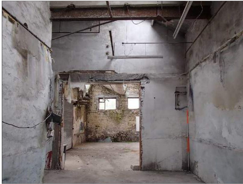
Plate 52 (shot 426): Former flywheel house showing later partition and doorway, looking east-northeast, 2m scale
