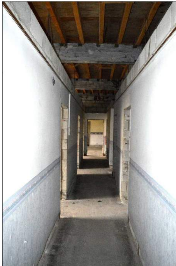
Plate 38 (shot 96): Corridor in the centre of the ground floor. Looking east, 1m scale
