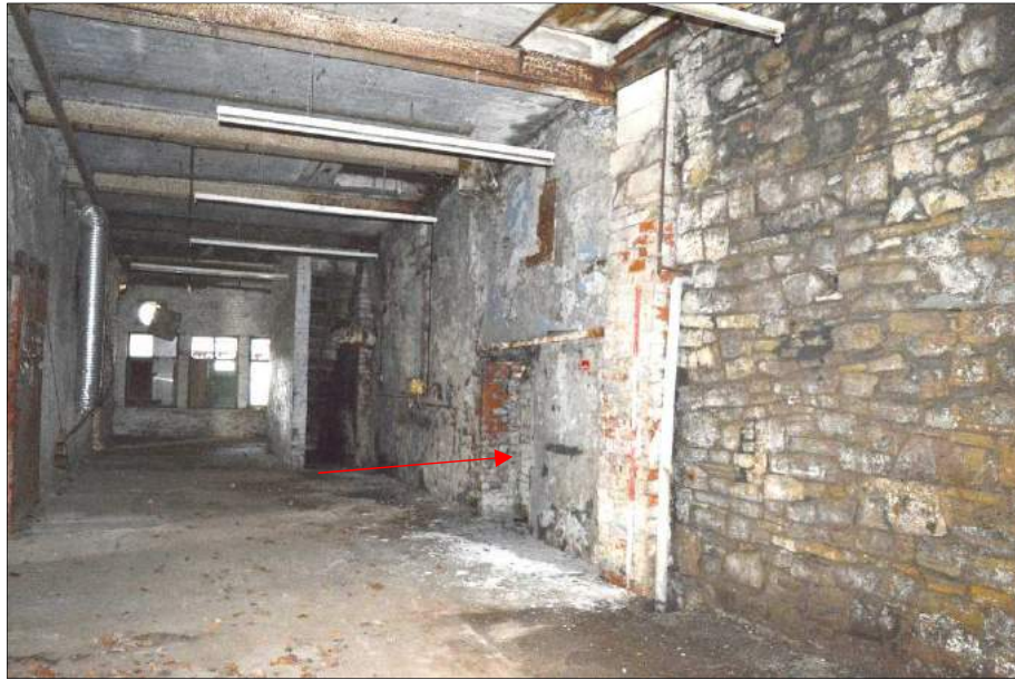
Plate 20 (shot 289): 1933 corridor looking towards the former 1908 lavatories to the east, potential hoist hatch in the ceiling in the foreground. Arrow points to bricked up opening. Looking east-northeast, 2m scale.
