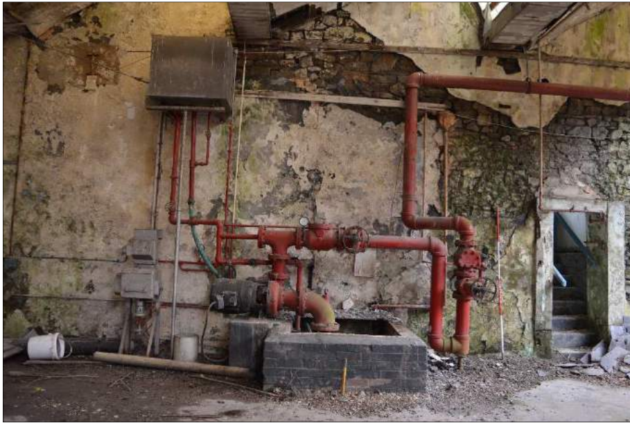
Plate 92 (shot 182): Water pump system by Mather & Platt. Looking southwest, 2m scale
