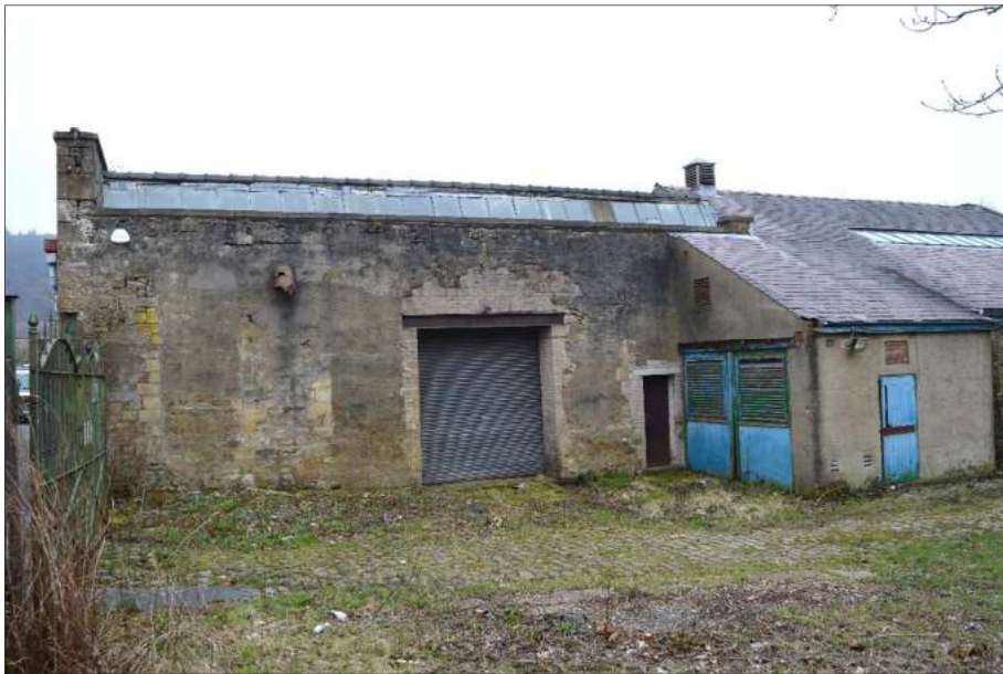
Plate 45 (shot 47): Former engine house with blocked up windows to the left and later square opening to the right. Looking southeast
