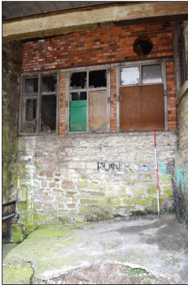
Plate 9 (shot 398): The 1908 WC extension on the southwest corner of Building A. Looking west-southwest, 2m scale
