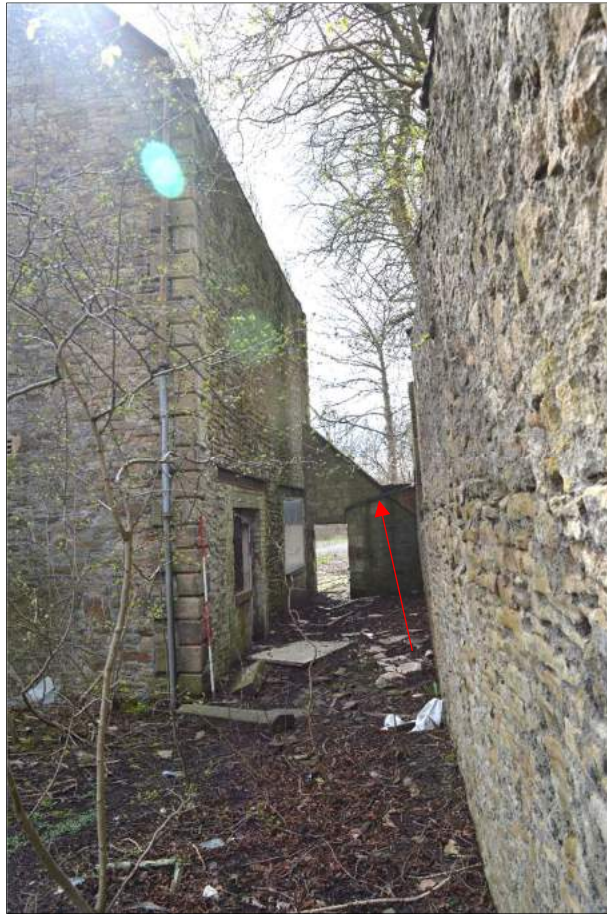
Plate 6 (shot 389): North elevation of the 1933 extension to the left and the boundary wall to the right. Arrow points to remains of roof of demolished lean-to. Looking southwest, 2m scale
