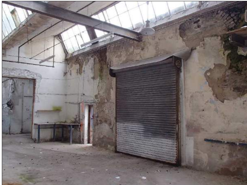
Plate 51 (shot 419): Brick arches revealed under render on the north wall. Looking northwest, 2m scale
