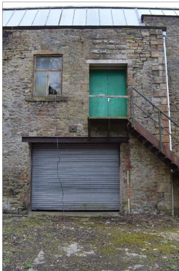
Plate 4 (shot 380): Blocked opening on first floor and new square entrance on ground floor. Looking southeast, 2m scale
