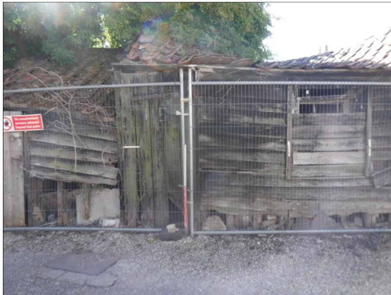
Plate 32 (shot 29): General view of southwestern part of northwest elevation showing poor condition. Looking southeast, 1m scale
