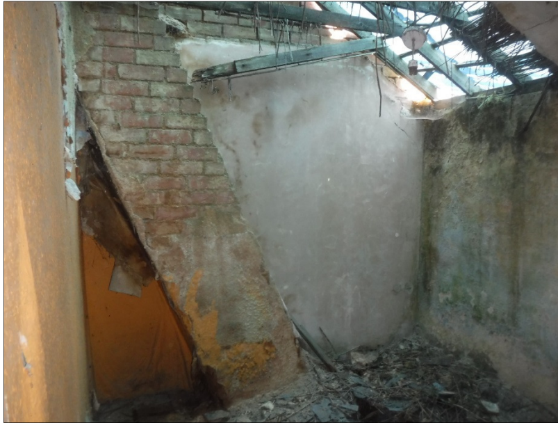
Plate 16 (shot 68): Dilapidated roof and ceiling. Chimney breast in light red coloured bricks. Looking north
