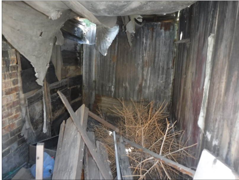
Plate 35 (shot 37): Internal view showing corrugated steel on rear wall and brick partition. Looking southeast
