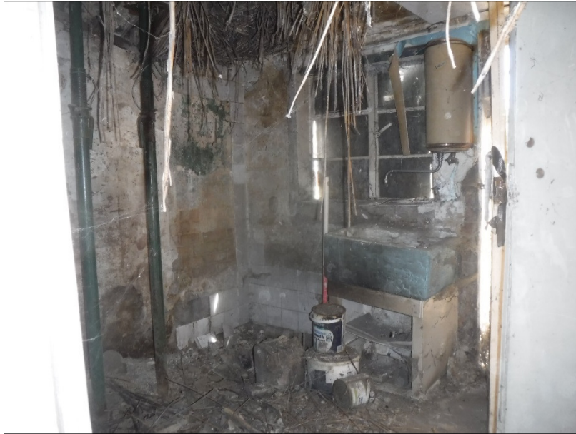
Plate 14 (shot 65): Dilapidated kitchen of No 115. Looking north, 1m scale
