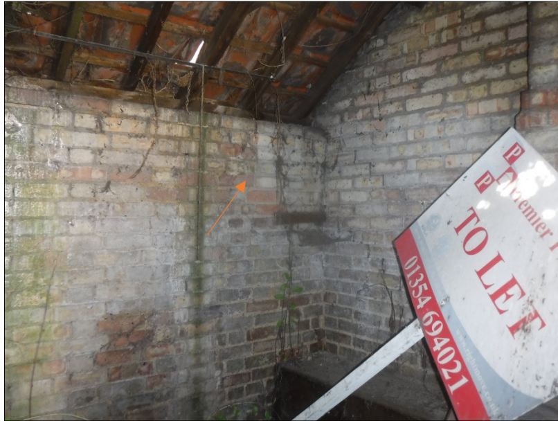
Plate 23 (shot 11): Southeast elevation with monk bond and arrow pointing to possible bricked up opening. Looking south
