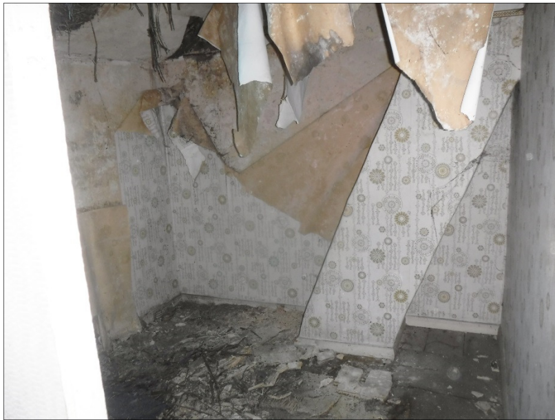
Plate 10 (shot 59): Small bedroom to the rear in 113 showing chimney flue. Looking southeast
