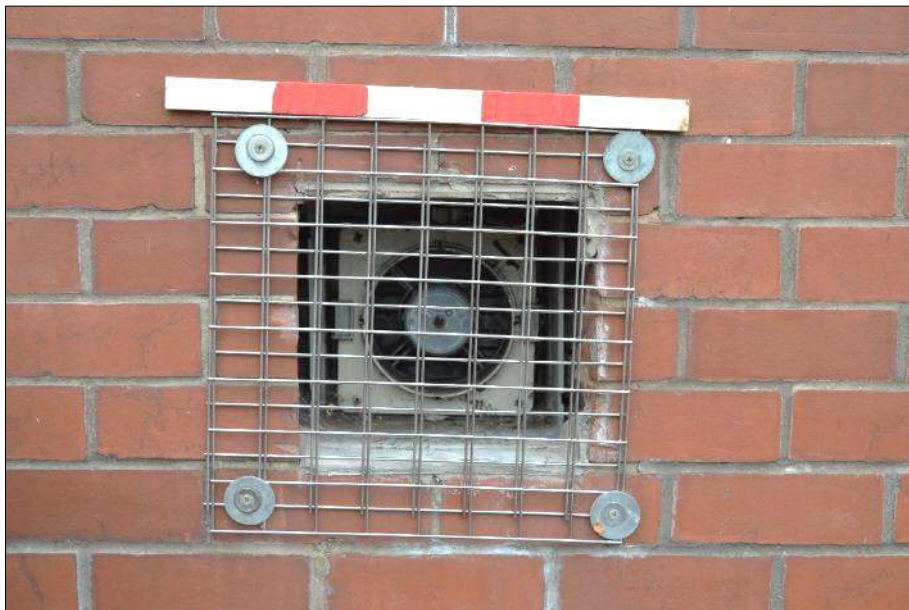
Plate 23 (shot 34): Air vent in south elevation of 1960's extension looking north, scale 0.5m
