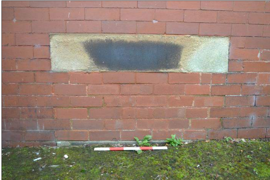
Plate 12 (shot 55): Sandstone lintel in original buildings north elevation looking south, scale 0.5m
