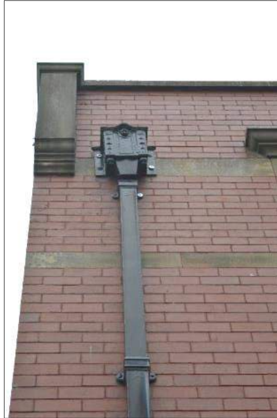
Plate 7 (shot 6): Cast iron hopper and downpipe on west facing elevation, looking east
