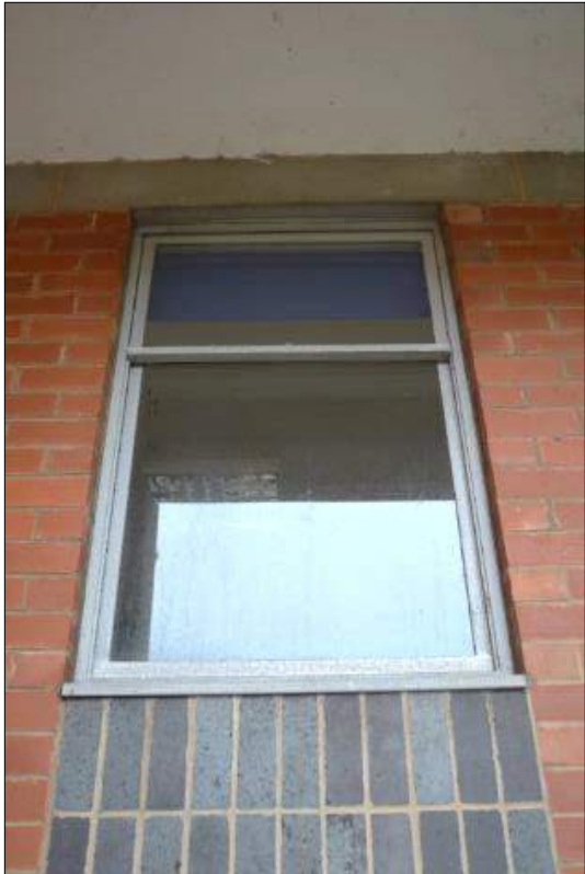
Plate 17 (shot 20): Ground floor window in west elevation of 1960's extension, looking east
