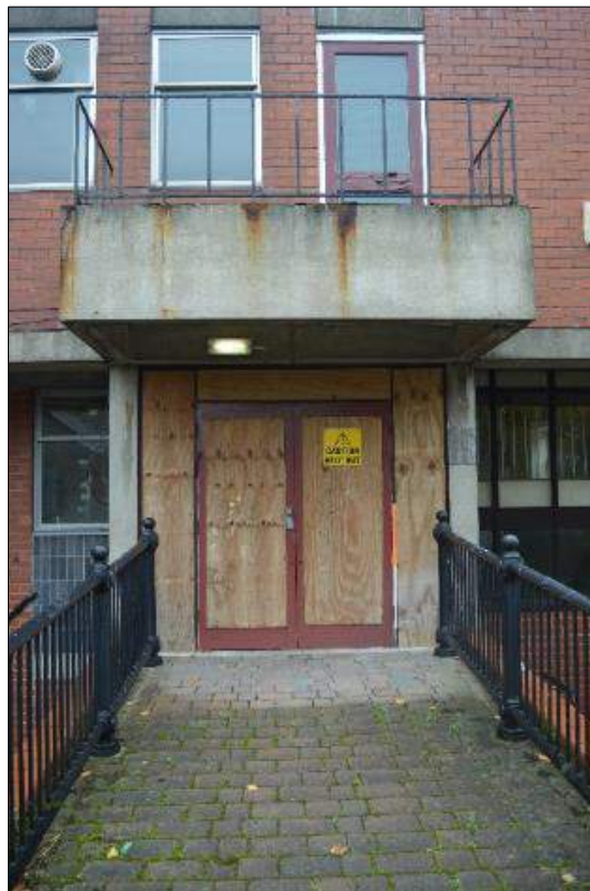
Plate 14 (shot 17): Main entrance to west elevation of 1960's extension looking east, 1m scale
