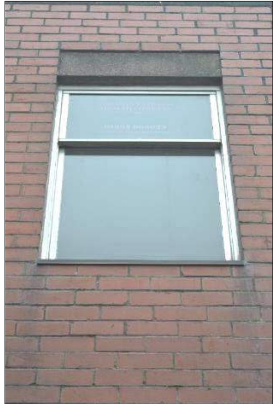
Plate 18 (shot 21): First floor window in west elevation of 1960's extension, looking east
