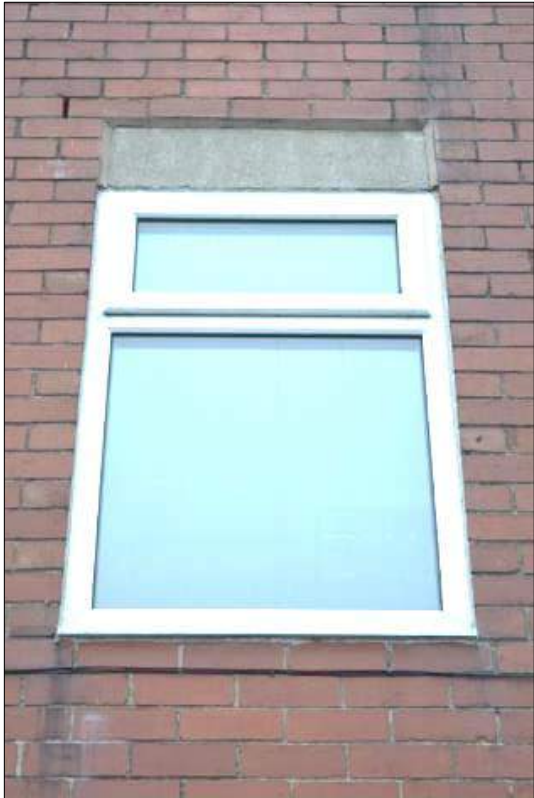
Plate 26 (shot 44): Ground floor uPVC window within east elevation of 1960's extension, looking west
