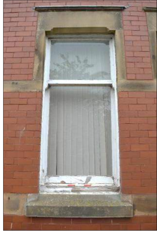
Plate 6 (shot 4): Ground floor window detail on west elevation looking east, 0.5m scale
