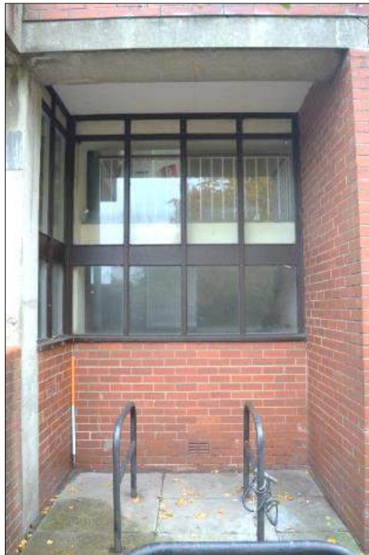
Plate 19 (shot 25): Bicycle parking bay in west elevation of 1960's extension looking east, 1m scale
