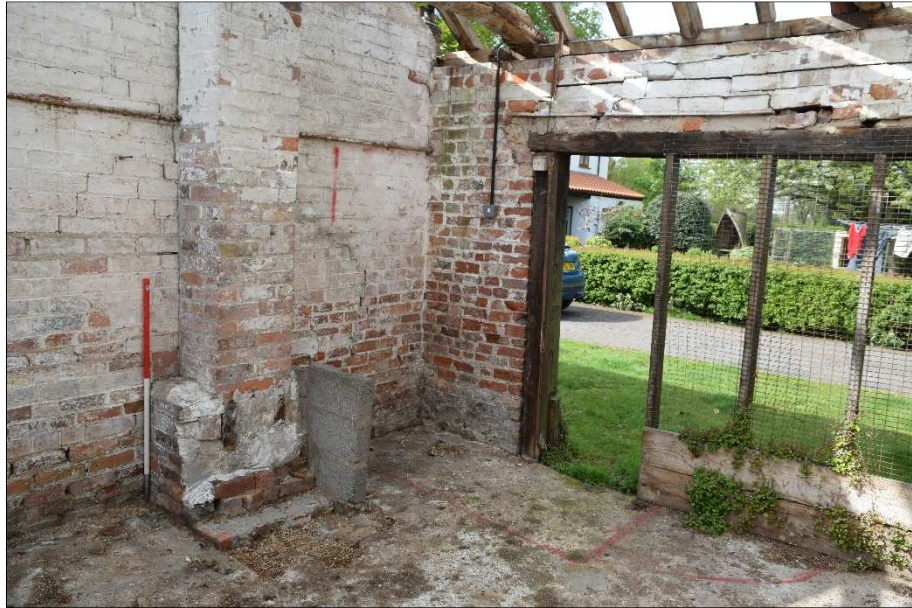
Plate 23 (shot 43): General view of former harness room with partially removed fireplace. Looking southwest, 1m scale
