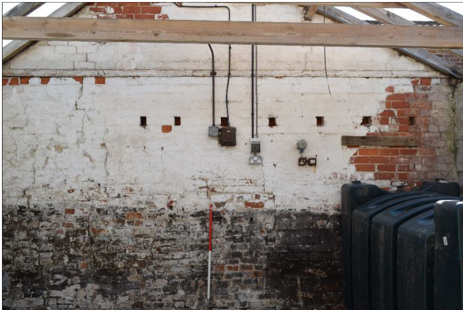
Plate 31 (shot 24): Holes on the east wall from removed fixtures
