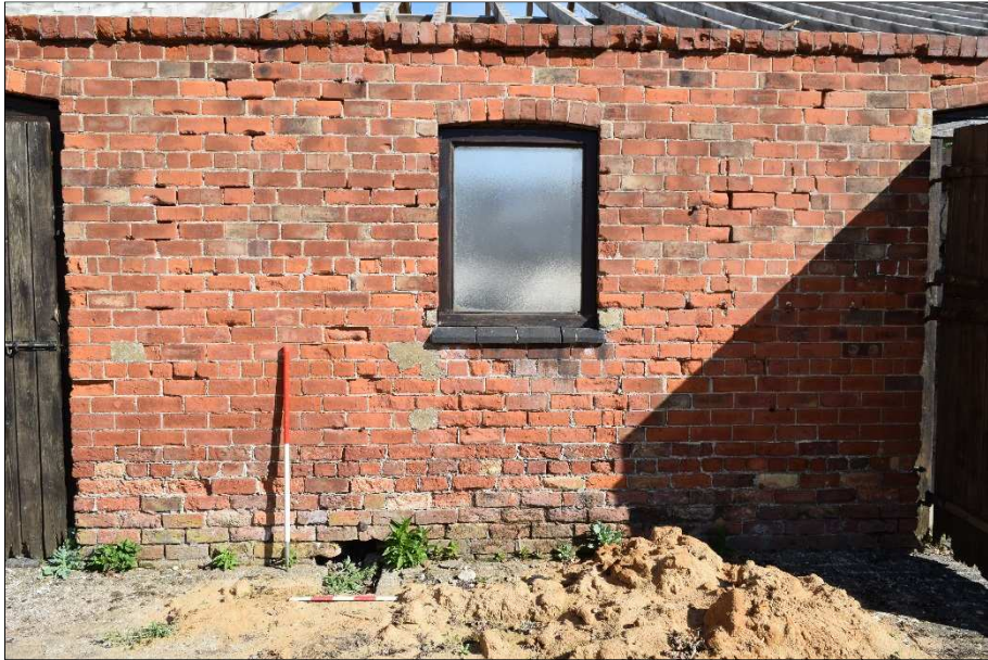
Plate 28 (shot 20): Close up of window and outlet of drain from the stable. Looking north, 1m scale
