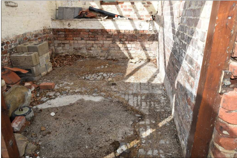
Plate 19 (shot 46): Worn floor surface in the northern stable box. Looking west
