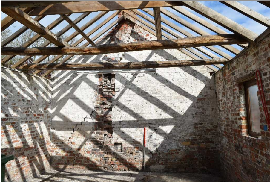
Plate 25 (shot 47): General view of the southern bay showing partially removed chimney flue. Looking north, 1m scale
