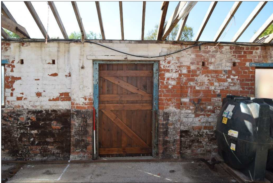
Plate 33 (shot 27): Representative stable door and removed saddle-tree fixtures on the wall. Looking south, 1m scale
