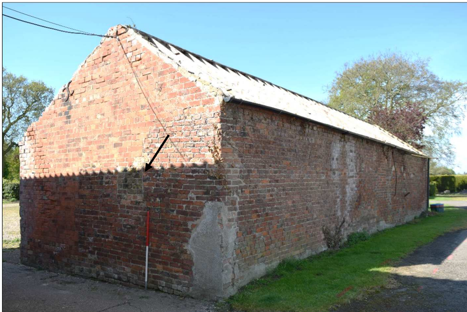
Plate 29 (shot 22): East elevation of Building B, with arrow pointing to possible blocked window. Looking southwest, 1m scale
