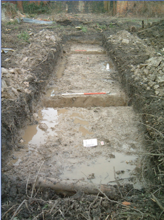
Plate 1: Trench 1, with slots excavated through natural alluvium. Looking north from south end of trench
