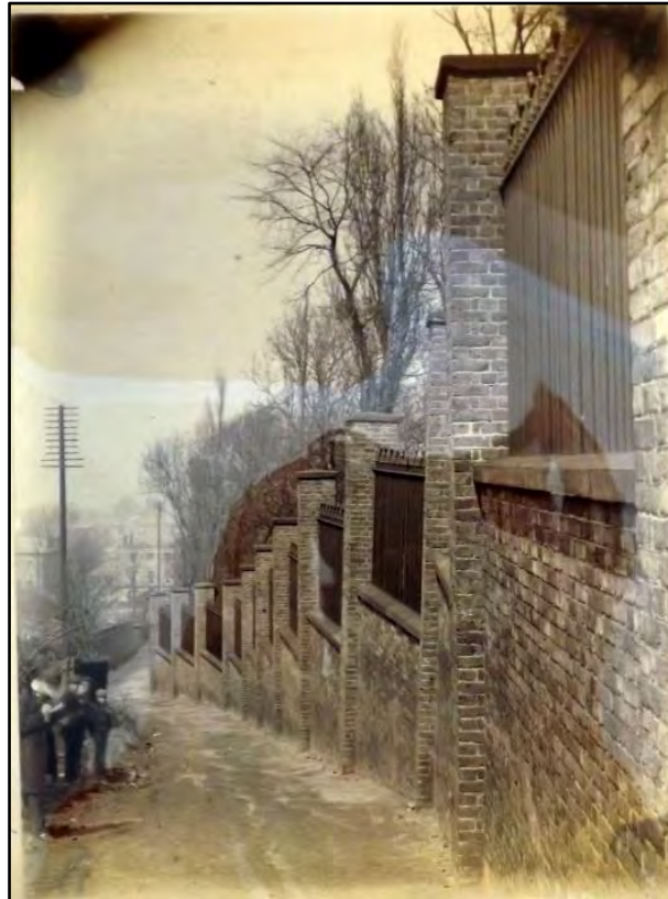
Plate 2: Boundary wall on Cemetery Road, circa 1899, showing tilting brick pillars
