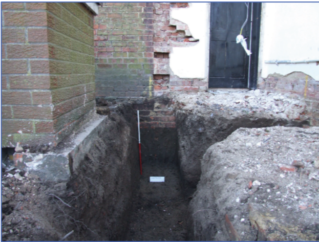
Plate 2: Footings of the existing school building exposed in the south-east corner of the development area. Looking south-south-west.
