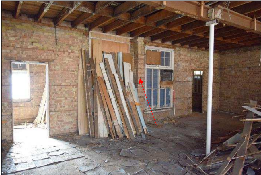
Plate 49 (shot 57): South wall of D, showing original window to the centre right and access to Extension F to the far right. Arrow points to former partition. Looking west, 1m scale
