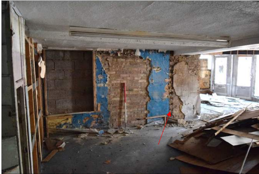
Plate 32 (shot 37): Blocked window next to a blocked doorway, behind the scale on the west wall, the arrow points to a removed partition where the blue painted plaster ends. Looking northwest, 1m scale
