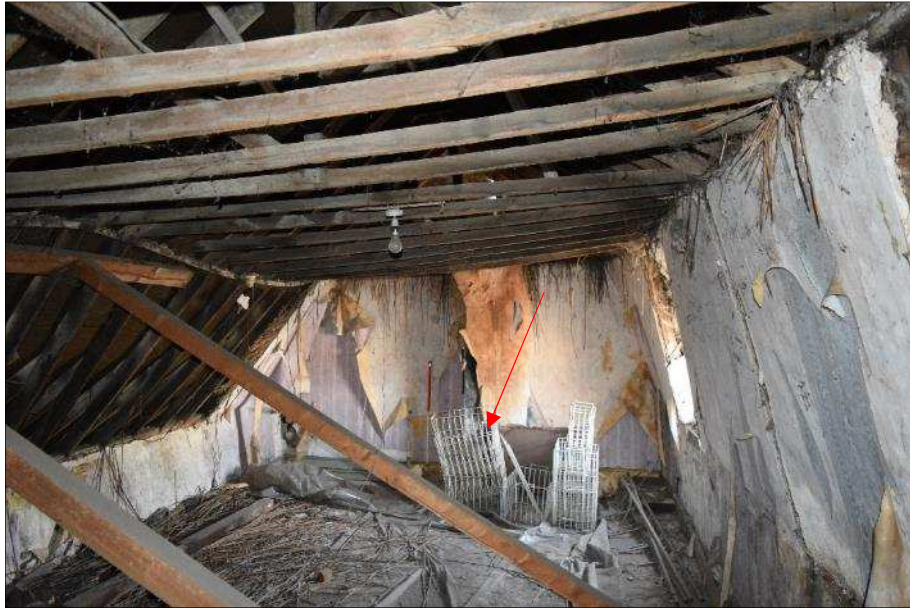
Plate 15 (shot 28): General view towards the partition wall, arrow points to a boarded-up fireplace. Looking south-southeast, 1m scale
