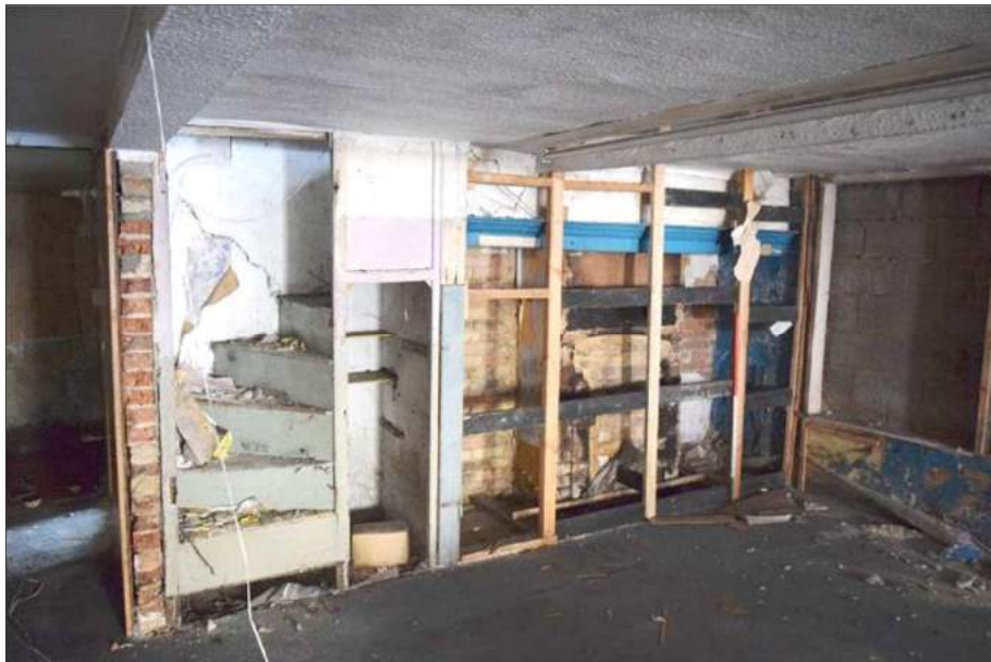
Plate 31 (shot 35): South partition wall showing original staircase, under-stairs cupboard and bricked-up fireplace behind modern stud wall. Looking southwest, 1m scale
