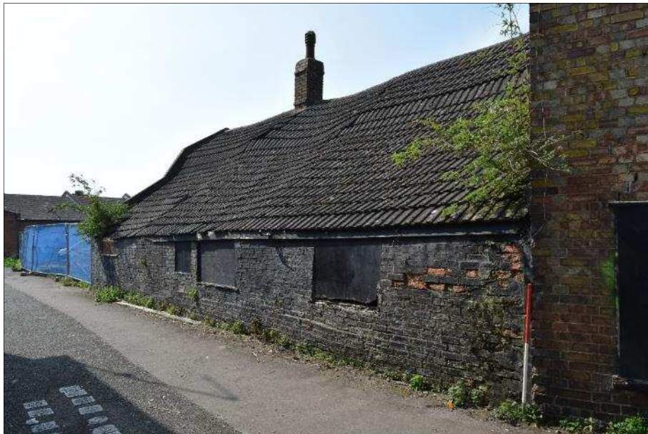
Plate 4 (Plate 80): East elevation, showing four boarded up openings on extension B. Looking southwest, 1m scale
