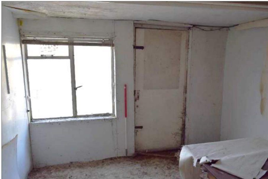
Plate 21 (shot 16): General view of the ground floor southern room. Looking west-northwest, 1m scale
