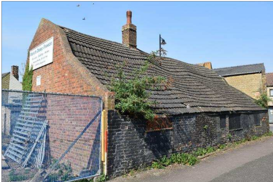
Plate 3 (shot 78): View of east elevation showing sagging roof. Looking northwest, 1m scale
