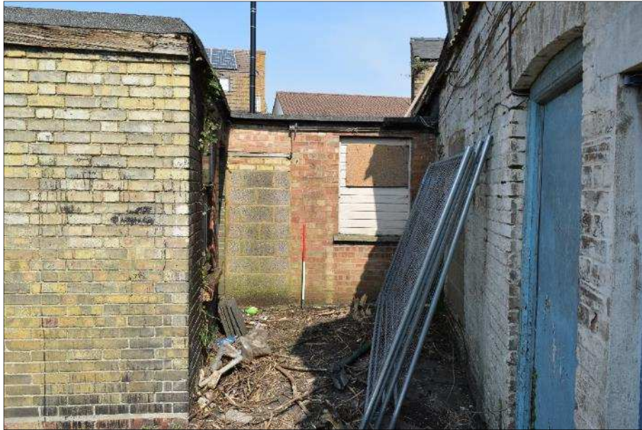
Plate 42 (shot 71): Blocked window and doorway on the south elevation. Looking north-northeast, 1m scale
