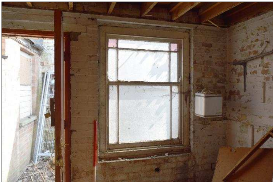
Plate 56 (shot 54): General view of east room in F. Looking southeast, 1m scale
