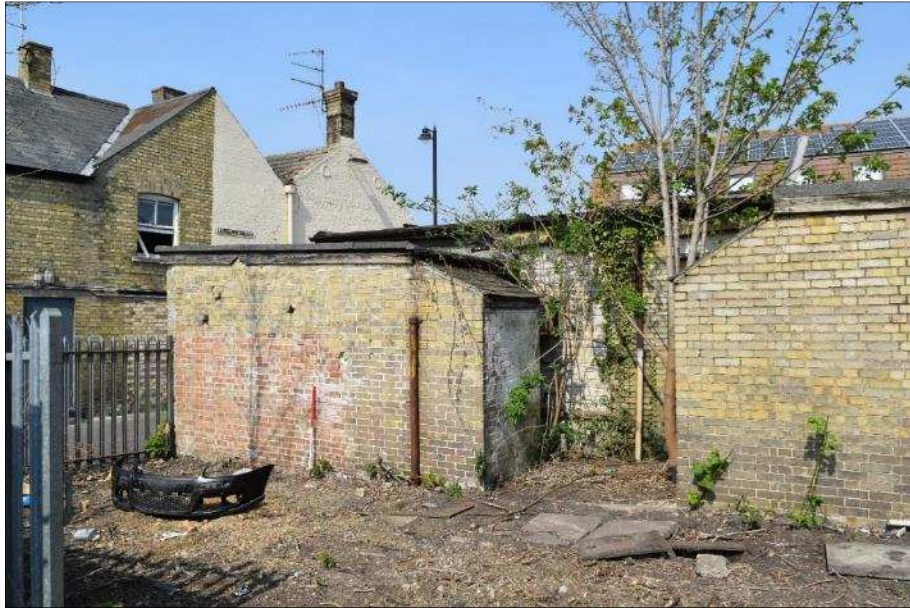
Plate 44 (shot 76): South and east-facing elevations of Structure E to the left. Looking north-northwest, 1m scale
