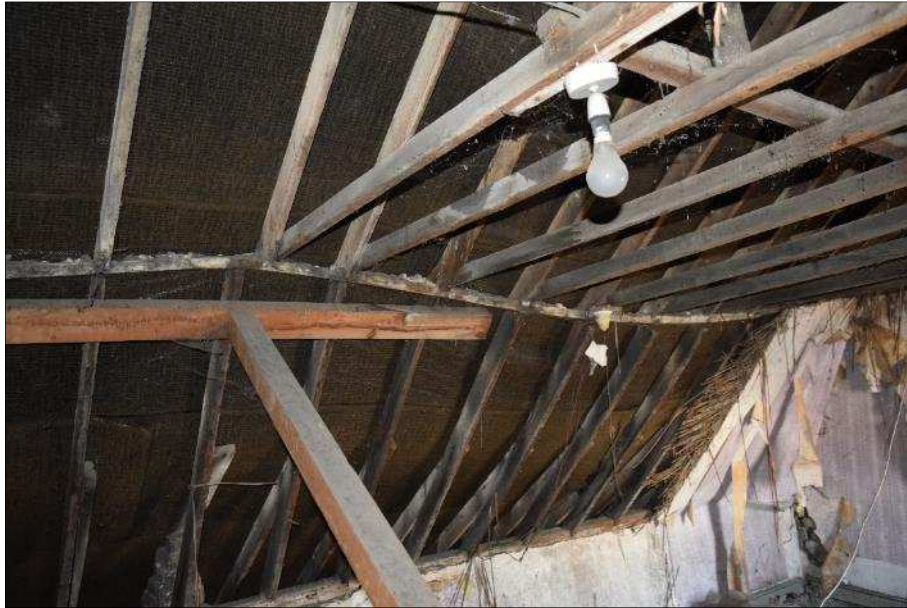
Plate 20 (shot 29): General view of poorly constructed roof. Looking south-southeast
