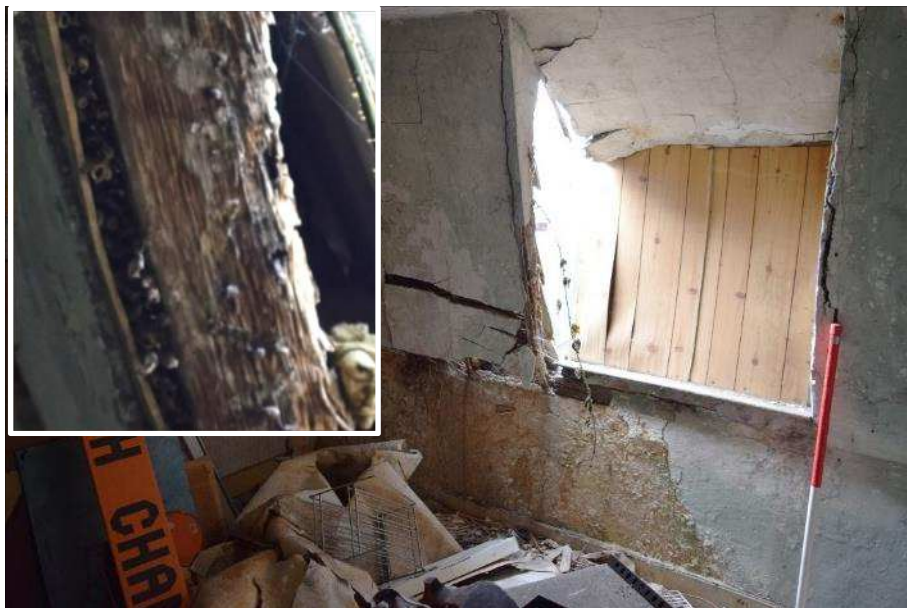
Plate 12 (shot 2): General view of boarded up dormer. Looking southeast, scale 1m. Inset shows reeds in situ adjacent to window
