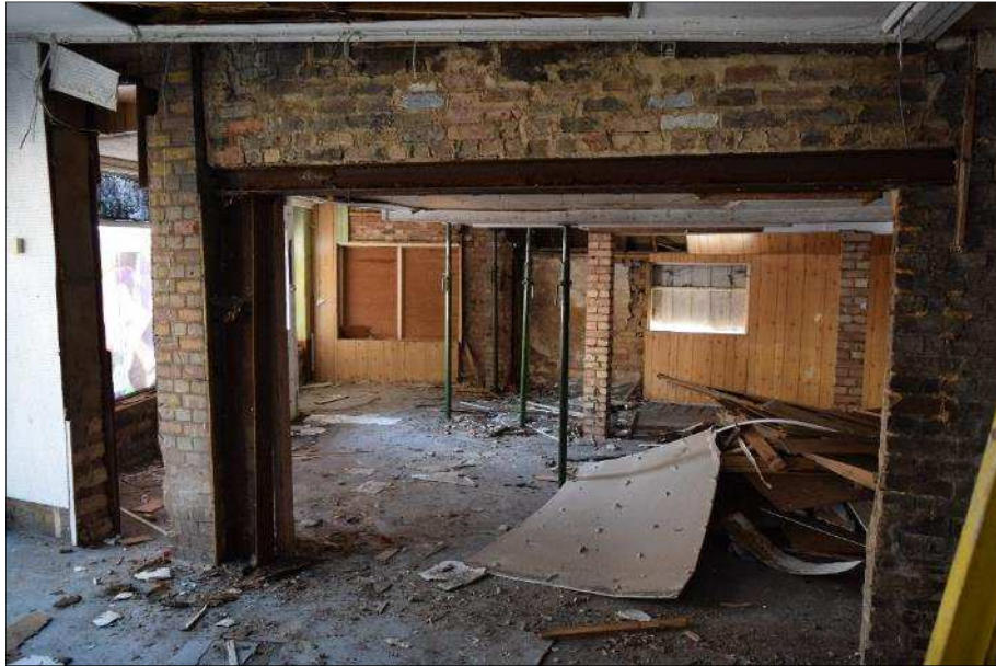
Plate 28 (shot 38): Large and later opening in the former west elevation of A. Looking northwest, 1m scale
