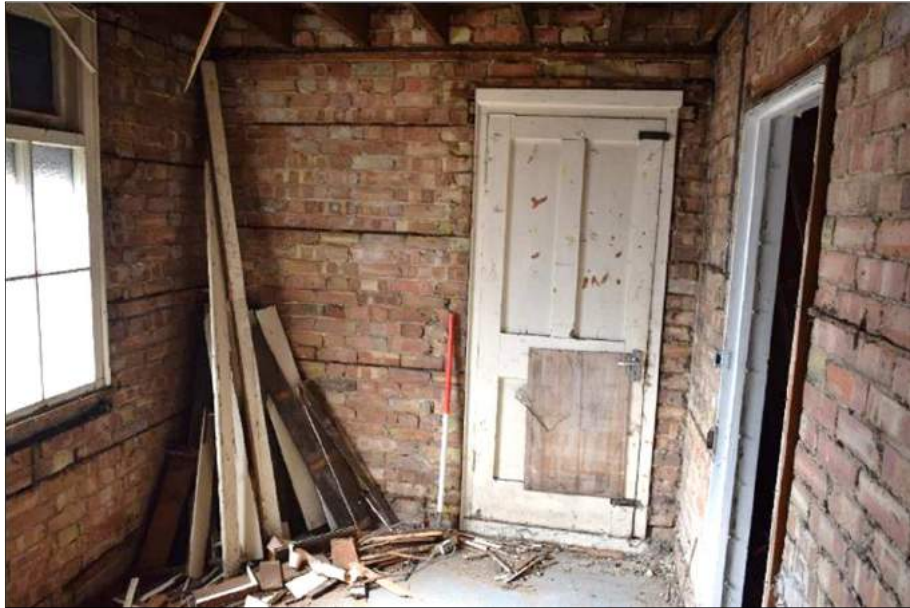
Plate 55 (shot 55): General view of Extension F looking west at the doorway leading to the yard. 1m scale
