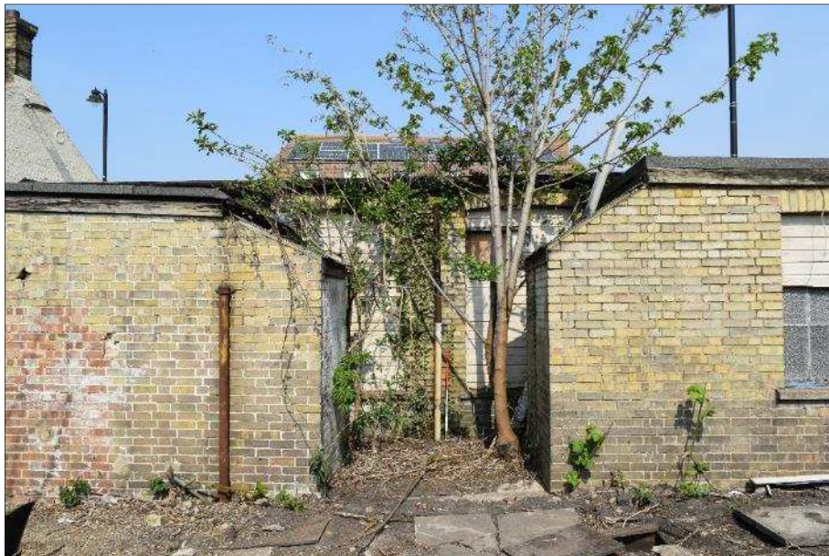
Plate 41 (shot 73): Largely obscured view of the south elevation of Structure D showing large blocked up segmental arched windows behind the tree. Looking north, 1m scale
