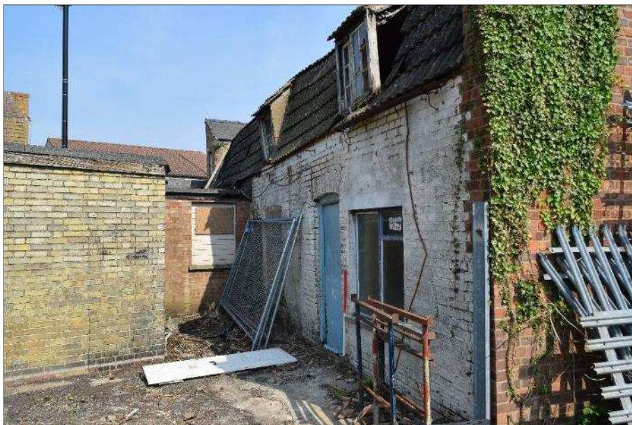
Plate 5 (shot 66): West elevation, abutted by later extension, two dormers on first floor. Structure A is abutted by Structure D. Yellow brick Extension E is visible to the left. Looking southeast, 2m scale
