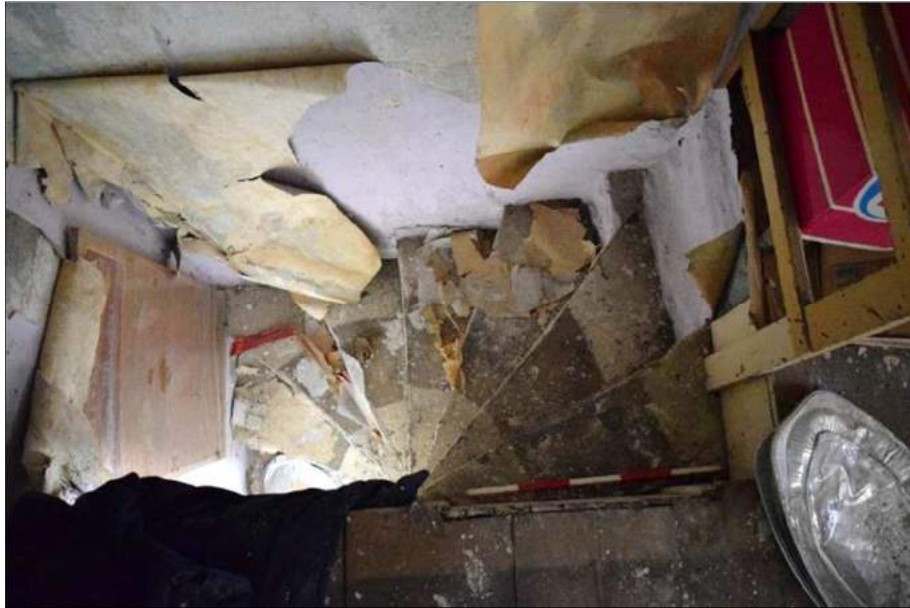
Plate 9 (shot 11): General view of winder staircase next to the chimneybreast. Looking south-southwest, 0.5m scale
