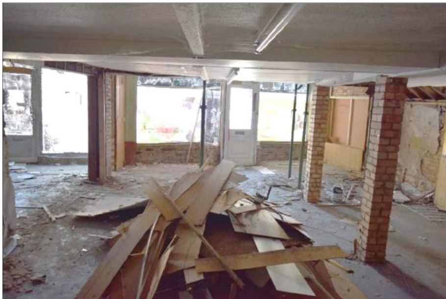
Plate 27 (shot 43): General view of north room merged with Structure C in the background and opening to Structure D to the left. Looking north-northeast, 1m scale
