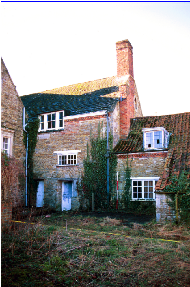
Plate 4: (013) The eastern elevations of the Eastern Range, detailing remodelling at the eaves and the insertion of dormers into the roof. Looking south-west.
