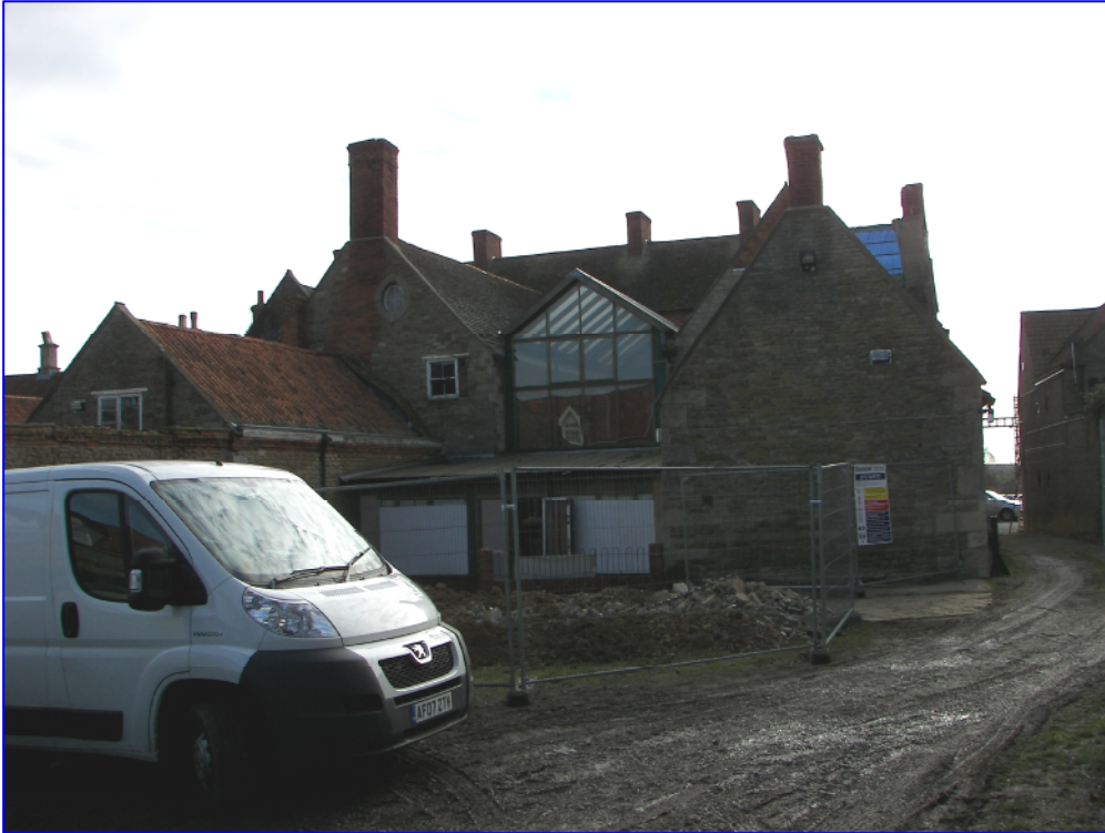
Plate 3: (178) Northern elevations showing the false garret bullseye window in the Eastern Range and the visually intrusive lean to abutting the atrium frame. Looking south-east.
