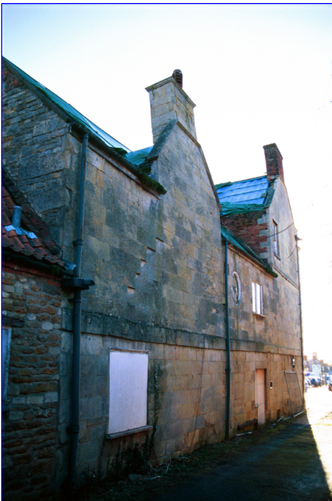
Plate 2: (009) The Western Elevation showing the ashlar cladding. Note the location of the Western Range stack behind the gable coping. The tarpaulin covers fire damage to the second floor. Looking south-east.
