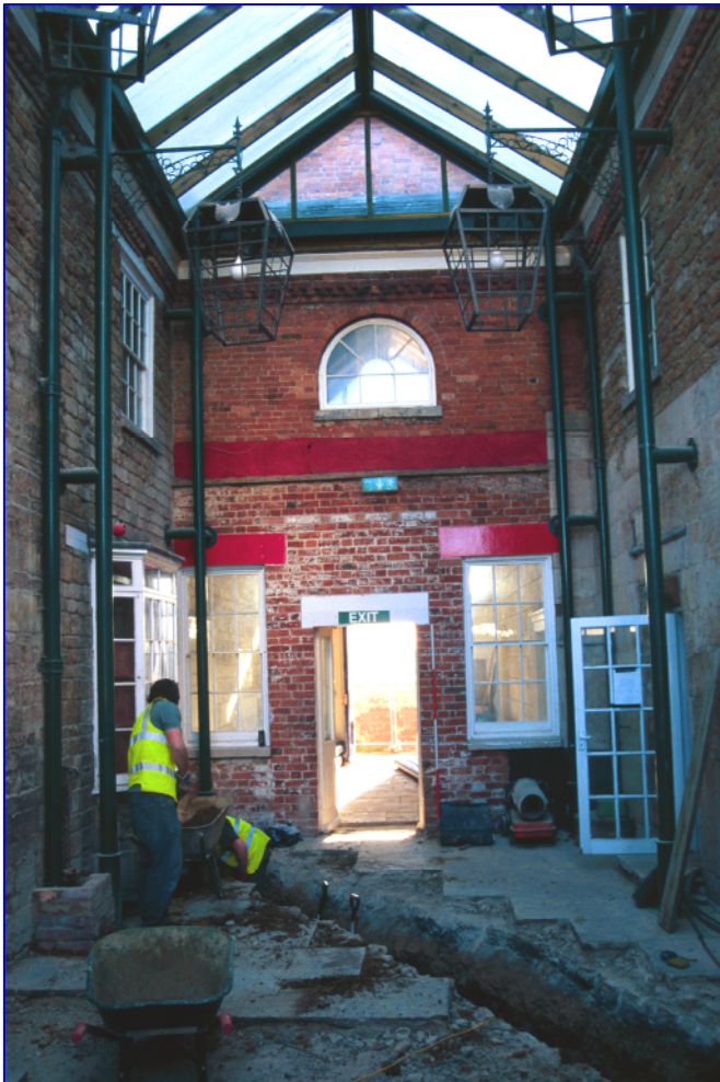
Plate 8: (027) Northern elevation of the carriageway arch with 19 th century infilling on the ground floor. Note the offset of the ashlar blockwork facia, in the right hand corner, necessary to correct the alignment between the Southern and Western Ranges. Looking south.
