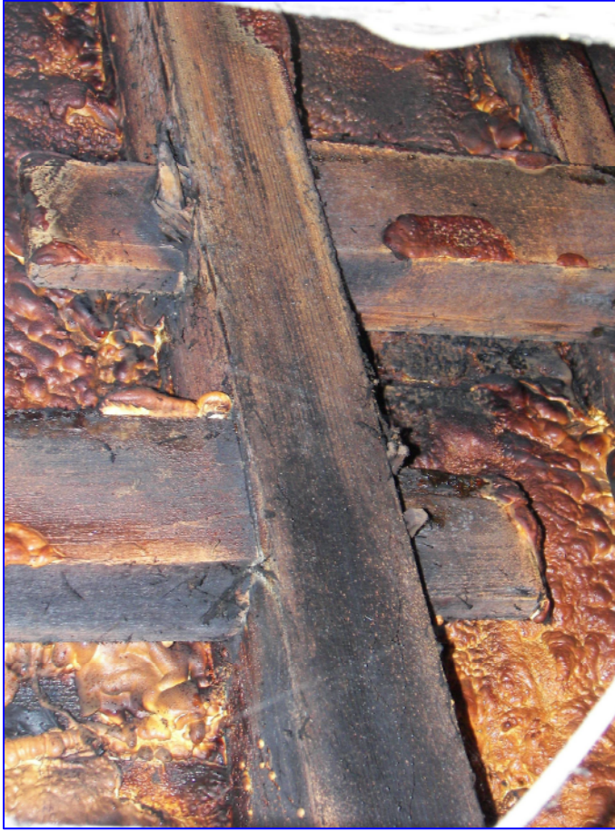
Plate 11: (shot 138) Staggered butt purlins morticed with tenons pegged behind the principal rafters and supporting common rafters. Observed in the fire damaged part of the Southern Range. Shot taken vertically.
