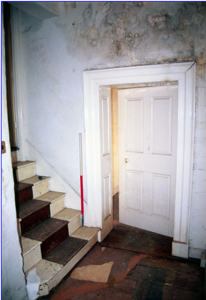
Plate 12: (074) On the first floor, rooms have doors that are four panel raised and fielded within a boxed, panelled frame with architrave. Shot depicts the door of Room 10 taken from the western half landing facing south.
