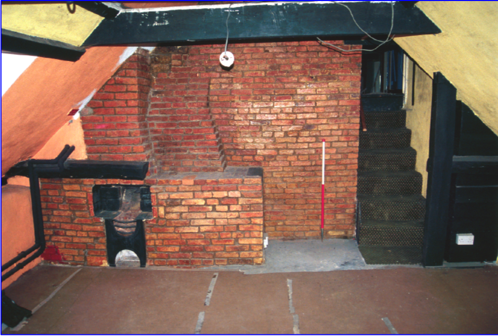
Plate 23: (083) Room 14. The southern wall is dominated by a large brick chimney breast that has a small hob grate built onto its eastern side. This structure also supports the stub end of a cross beam that has been cut to accommodate the insertion of stairs from Room 13. A timber stanchion at the foot of the stairs supports the opposing beam stub. Looking south.
