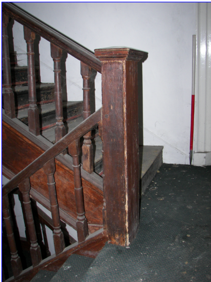
Plate 17: (167) The Western Range staircase, later 17 th /early 18 th century style, closed string construction with simple turned balusters, heavy plain handrail and balusters. Looking north.
