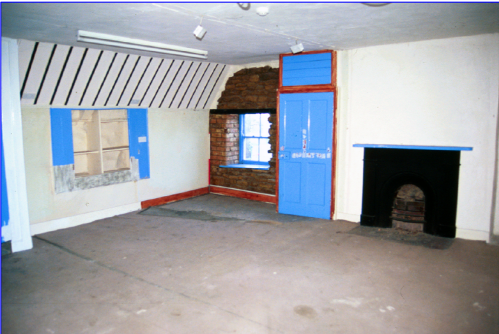
Plate 22: (079) Room 13, on the first floor of the Eastern Range. Set into the chimney breast on the northern wall is a 19 th century cast iron arched bath grate with a plain stone mantel and pillars. The door leads to Room 14 down a short flight of stairs. Looking north-west.
