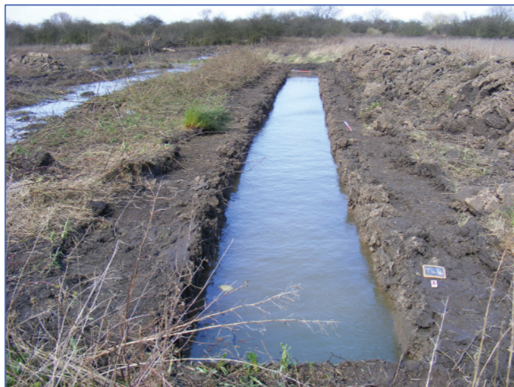
Plate 6: Trench 4, looking north from the south end of the trench, showing the impact of the high water table on the site.
