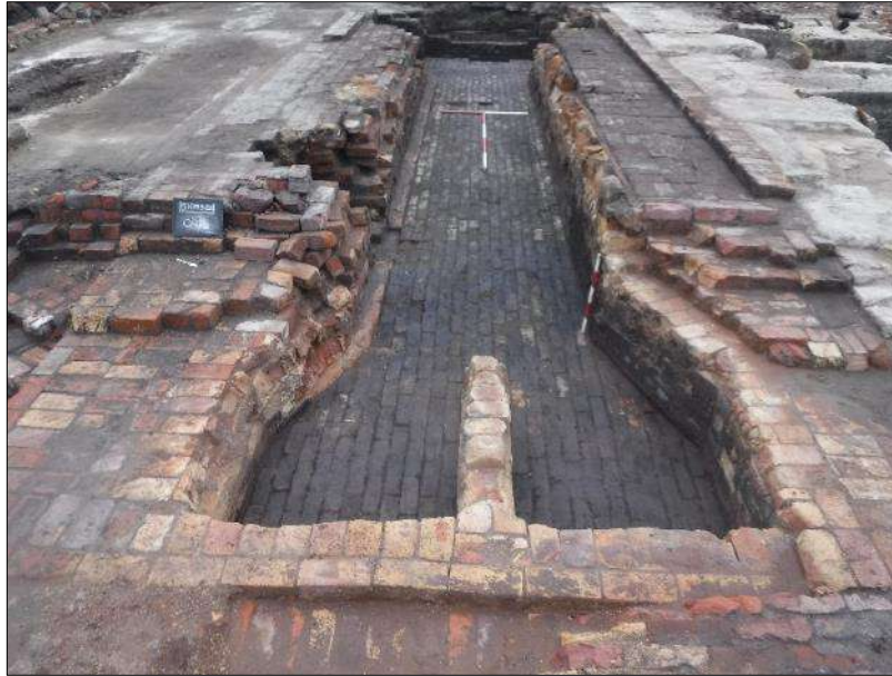
Plate 47: General view of Lancashire boiler base, looking southwest, 2m and 1m scales
