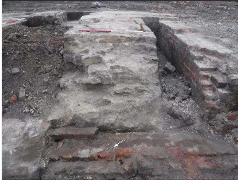
Plate 41: Masonry 178 within engine house showing fixing bolts in upper surface and wall 176 to the right, 1m scale
