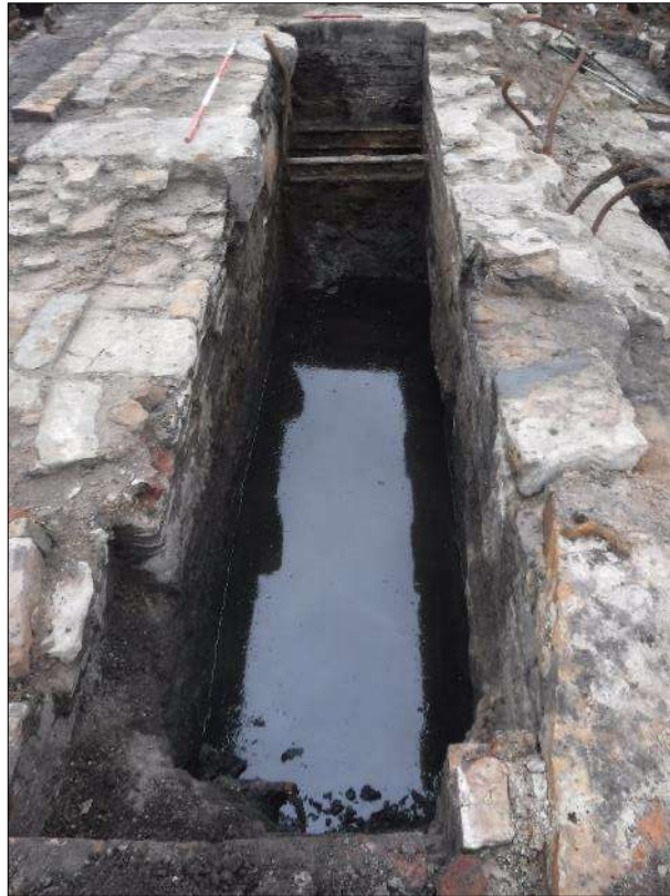
Plate 43: Pit between masonry 181 to the left and 183, 184 and 186 to the right, showing wrought iron joists and anchor bolts at southwestern end, looking southwest, 2m and 1m scales
