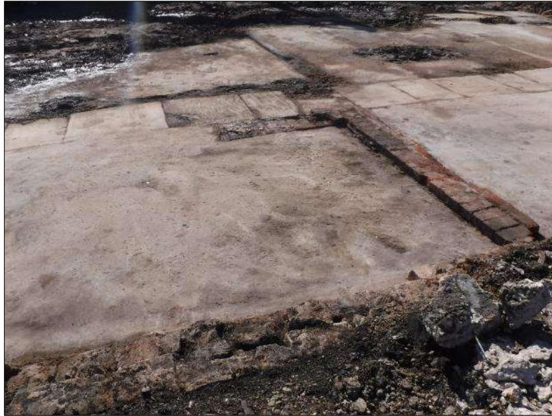
Plate 3: Brick partition wall 236 with sandstone wall 234 in foreground, showing central flagged surface 215 and later concrete floors, looking southwest, no scales
