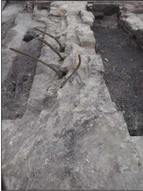
Plate 45: Masonry 183 within engine house showing fixing bolts in upper surface, no scale
