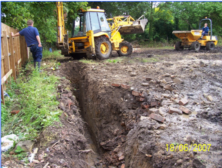
Plate 2: View along north side of Plot 1 footings, showing remains of former brick built soakaway. Looking east-north-east from north-west corner of the site
