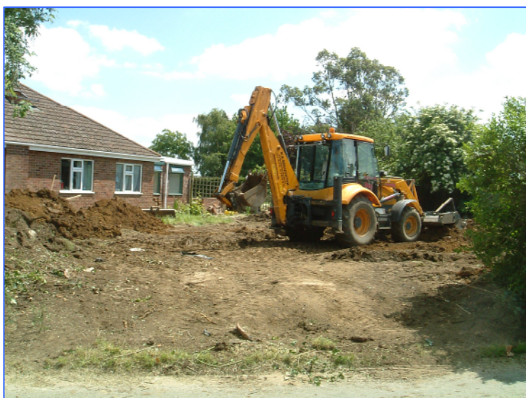
Plate 1: General view of the site looking south from the site entrance on Edenham Road.
