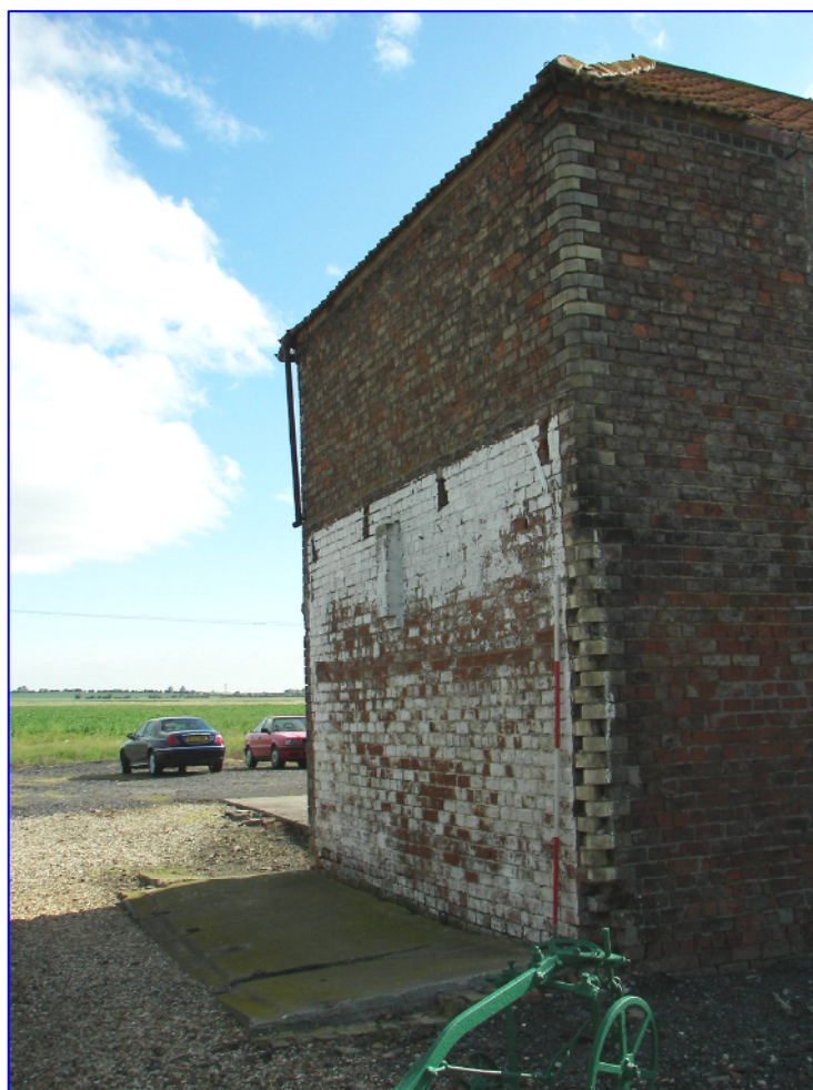
Plate 4 (Shot 9): The north-west facing elevation, looking north, showing the scarring from the recently demolished outbuilding and the surviving concrete floor.
