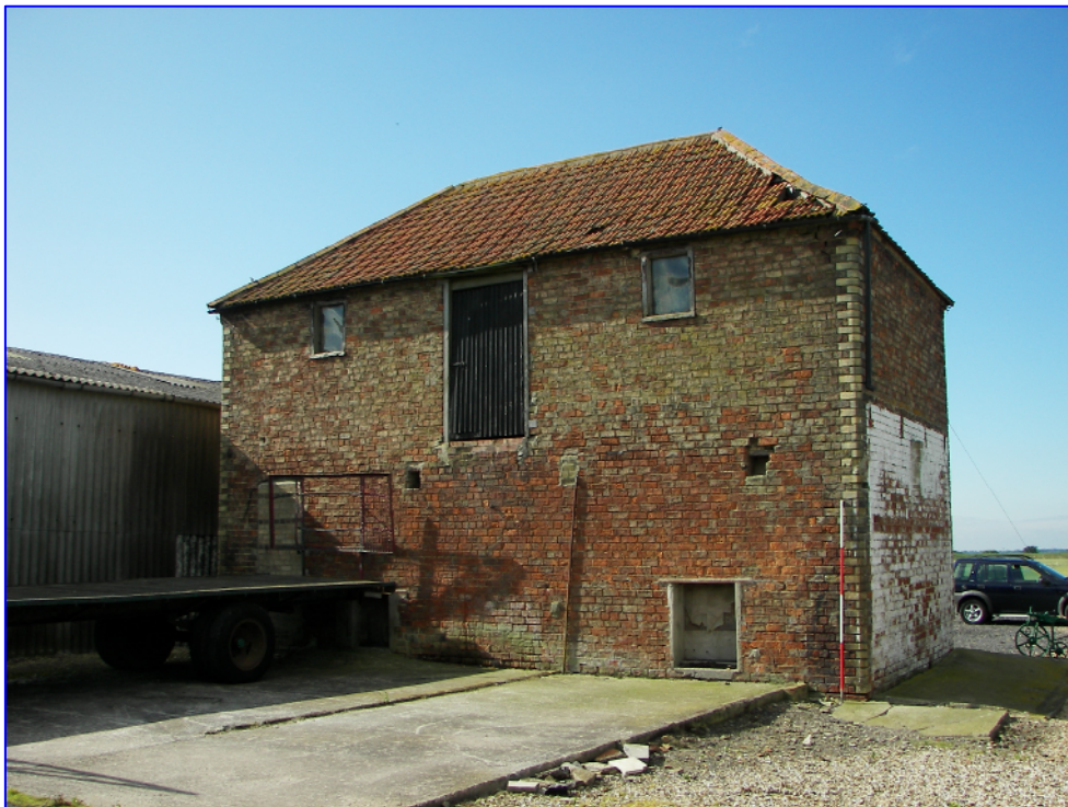
Plate 6 ( Shot 11): The north-east facing elevation viewed looking south. Note the concrete apron for the pig sties formerly accessed through the small openings in the barn wall.
