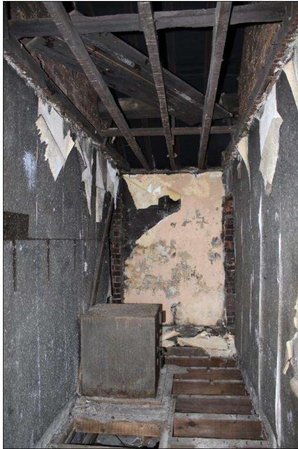
Plate 11 (shot 68): General view of box room and former landing/hallway with a potential blocked window, looking west
