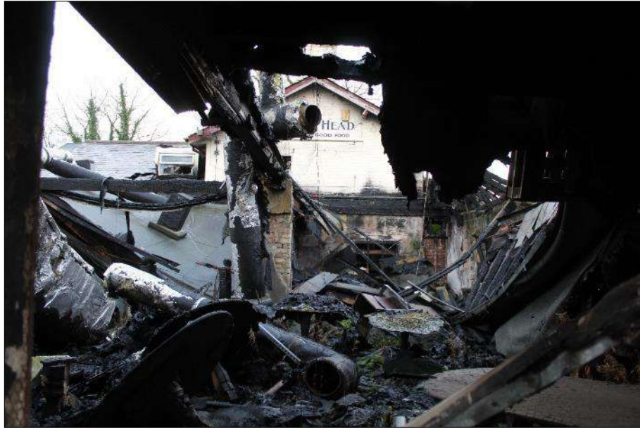
Plate 22 (shot 22): General view of the interior of the northern side of Structure C, looking south-southeast
