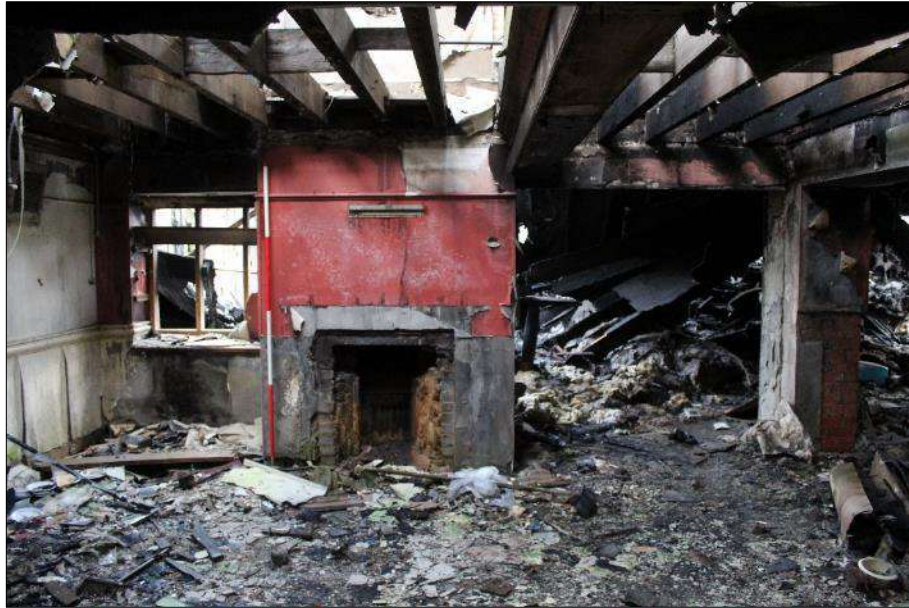
Plate 5 (shot 44): General view of interior of original structure, looking north, 2m scale
