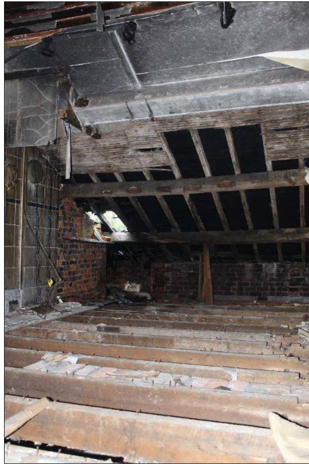
Plate 16 (shot 94): General view of the first floor of Structure B, looking northwest
