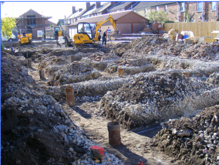
Plate 2: General view of Plots 2 – 5, showing the excavated ring beam foundations and the steel pile sleeves in situ. Looking west.
