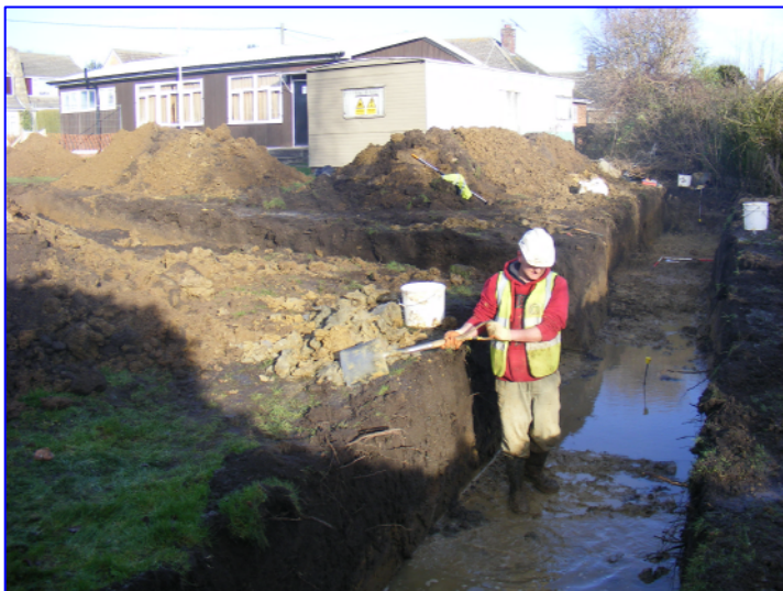
Plate 1: General site and working shot looking north, from the south-east corner of the site. Trench 1 is in the foreground, with Trench 2 to the left of the picture
