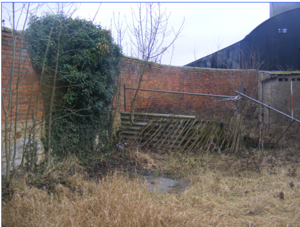
Plate 51 (Shot 103): Brick repair to west end of garden boundary wall, looking north-north-west.
