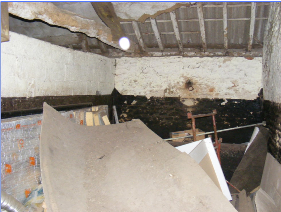
Plate 32 (Shot 11): Room D5, looking east-north-east, with brick partition to the left of the shot.
