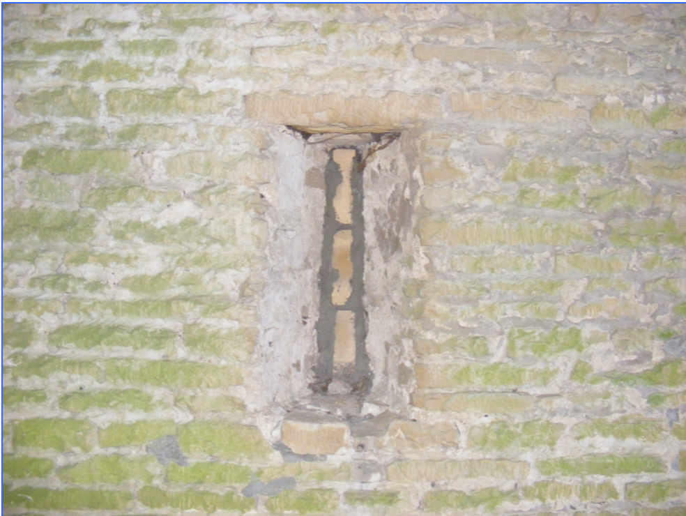
Plate 46 (Shot 113): Detail of blocked ventilation slit, internal east elevation of Building G, looking east-north-east.
