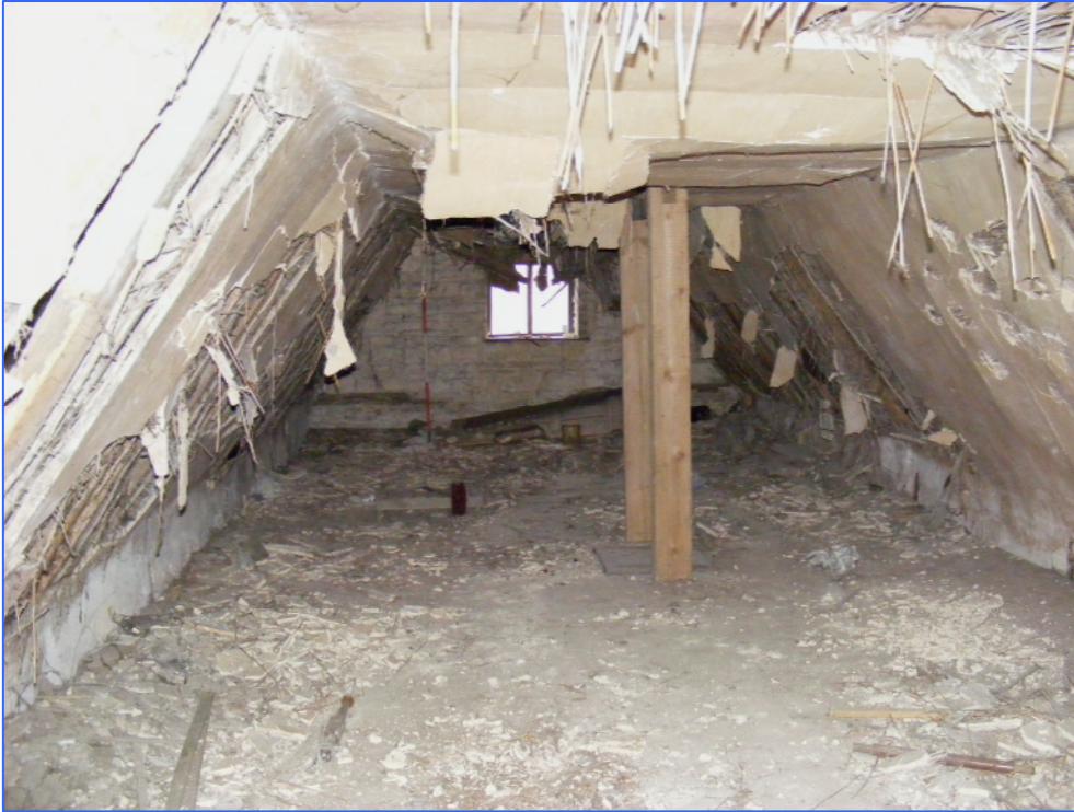
Plate 21 (Shot 52): Upper floor of Building B, looking east-north-east. In the centre of the shot is the hatch to the lower floor.
