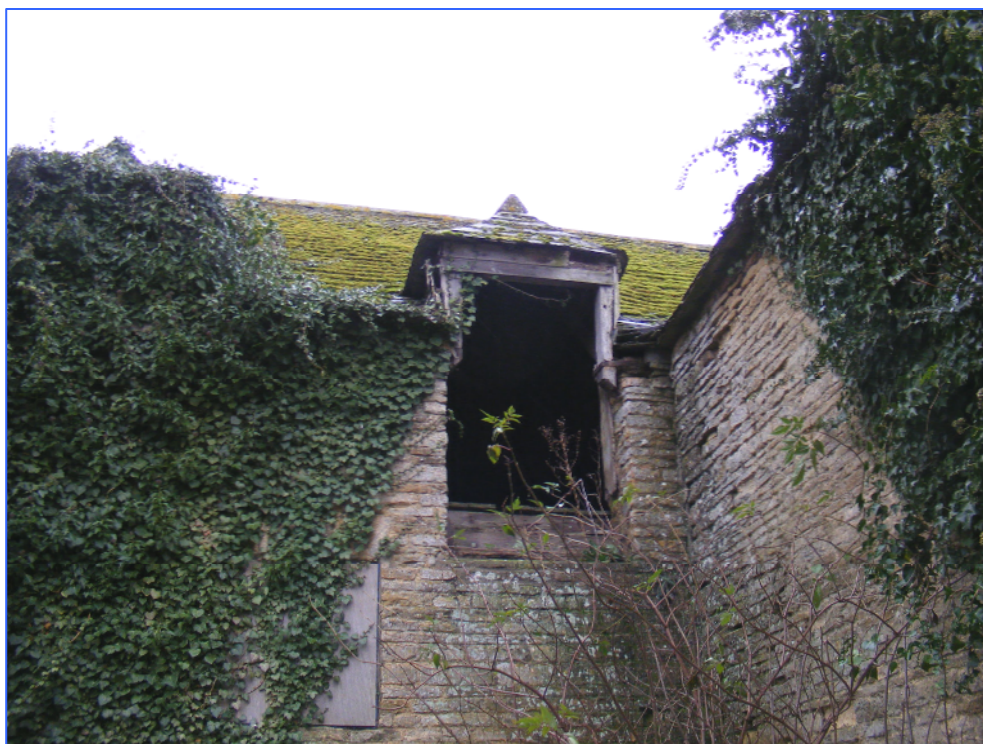
Plate 9 (Shot 95): Detail of doorway at north end of east elevation of Building A barn, looking west. The hipped roof reflects the design of the dormers on both this and the west elevation.
