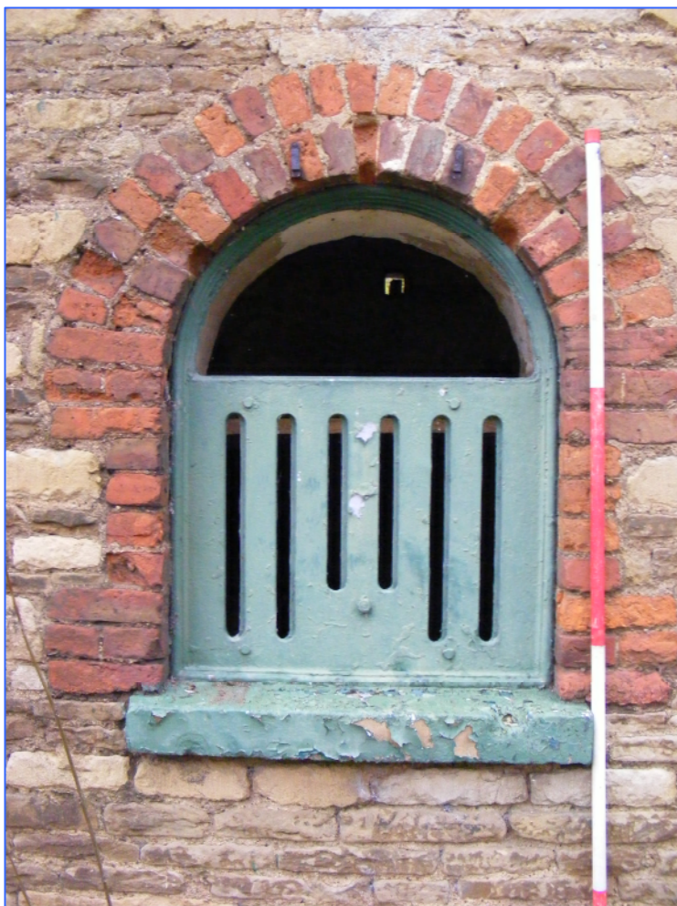
Plate 15 (Shot 43): Detail of ventilated opening in south elevation of Building B, looking north.
