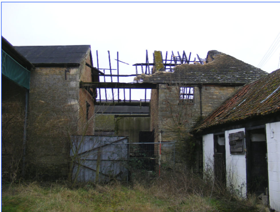
Plate 39 (Shot 60): East elevation of Building F, looking west-south-west, showing fire damage to the roof.
