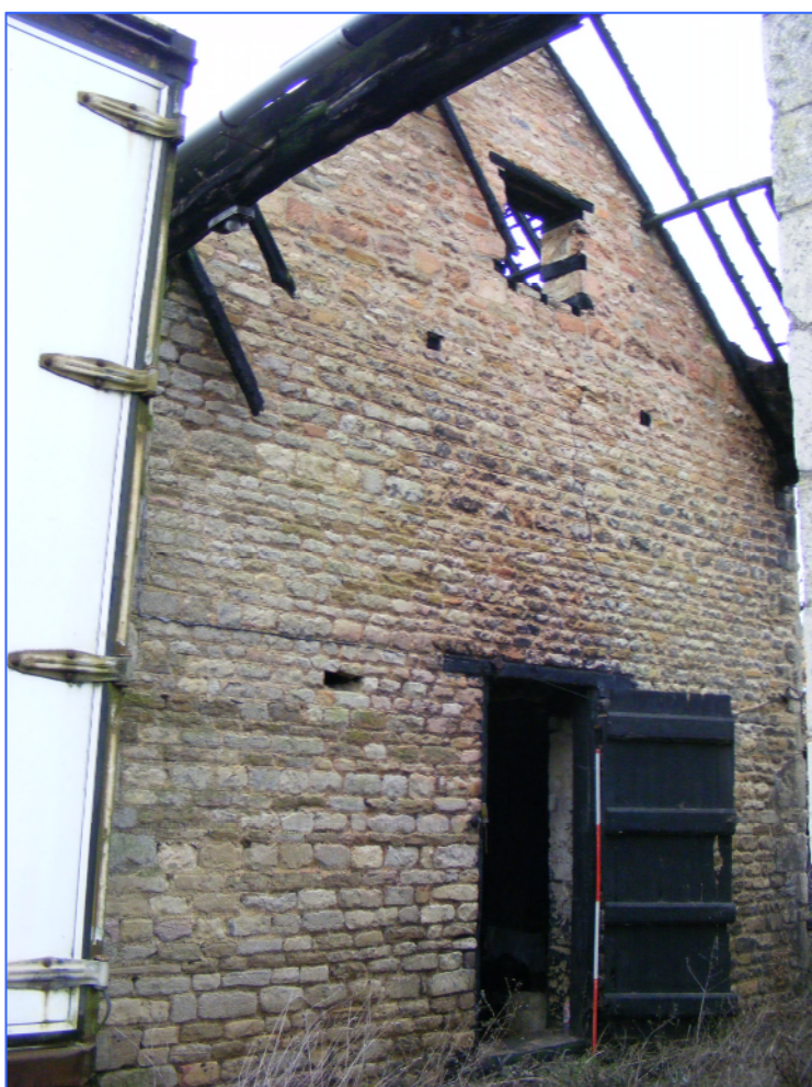
Plate 40 (Shot 67): South elevation of Building F, showing extent of fire damage, looking north-east.
