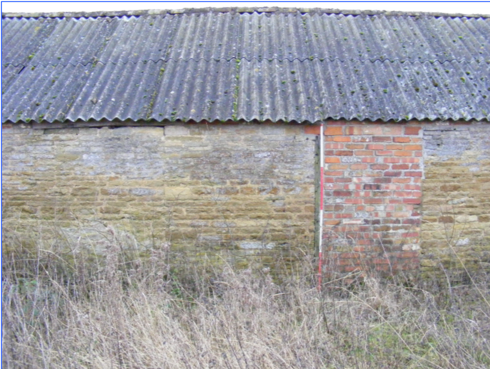
Plate 34 (Shot 32): Detail of blocked doorways in north elevation of Building E, looking south-south-east.
