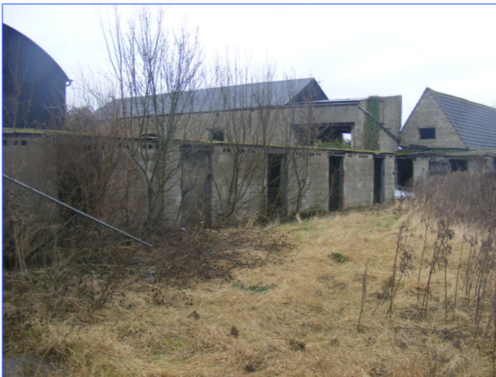
Plate 53 (Shot 102): Breeze block outbuildings along north side of walled garden, looking north-east, with Buildings G, H and B in the background.
