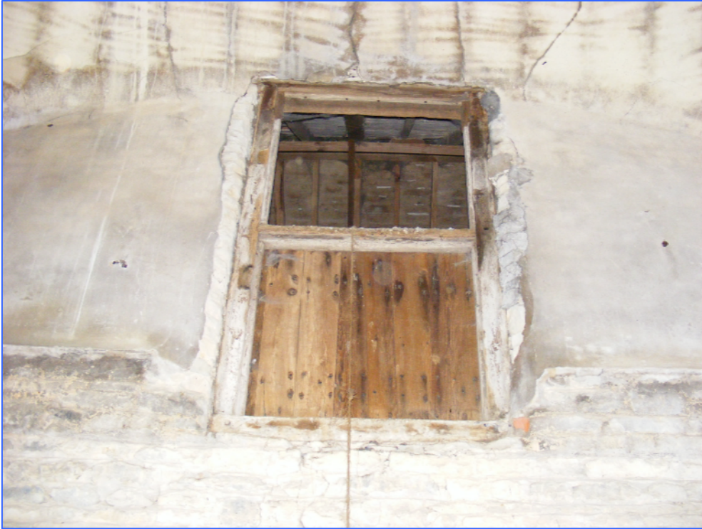
Plate 7 (Shot 83): Partially blocked doorway between the oast house and barn, looking west-south-west.
