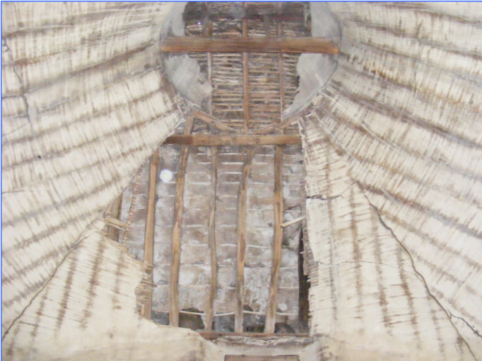
Plate 6 (Shot 77): Roof structure of oast house, looking north, showing area of recent collapse.
