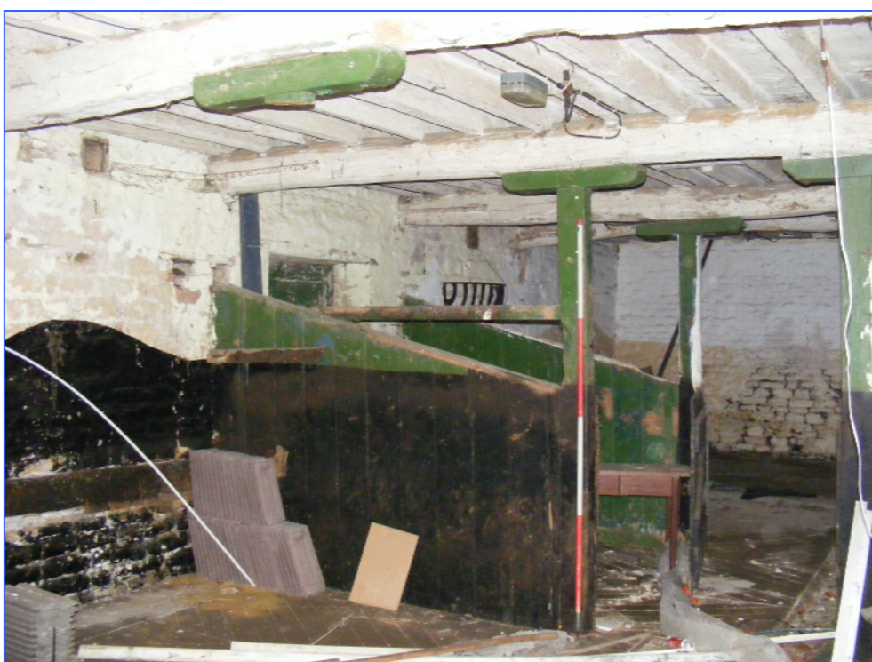
Plate 18 (Shot 48): Interior of stable block in Building B, looking east-north-east. Note the remnant of a former partition attached to the ceiling joist in the foreground.
