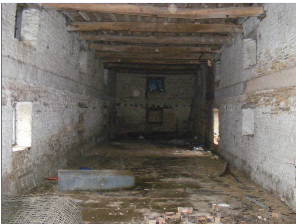
Plate 11 (Shot 74): Interior of Building A barn, looking north-north-west. Note the remnants of the former first floor joists at the far end of the building.
