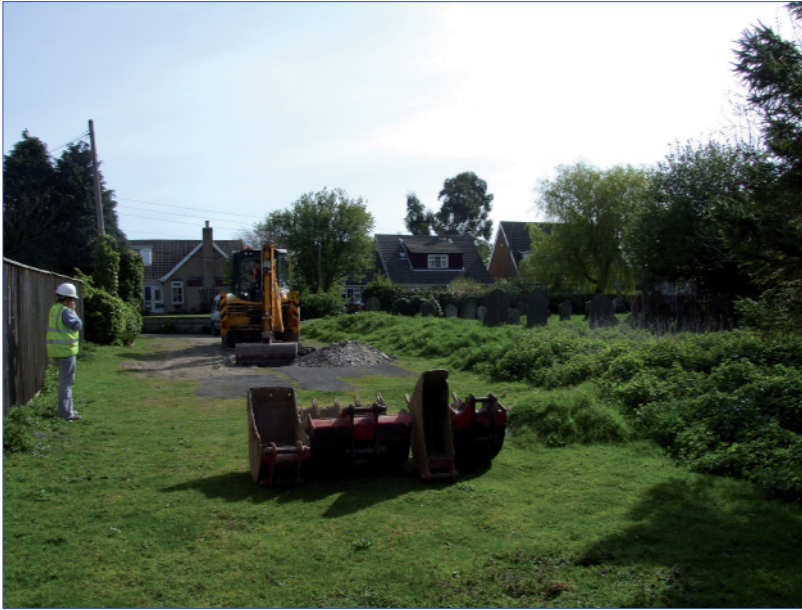
Plate 1: Overall site shot at start of machining taken to the west of the trench and looking east
