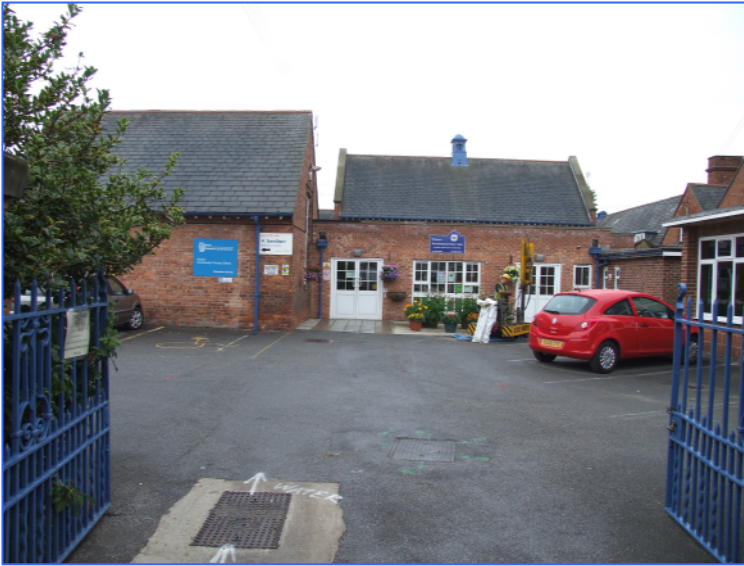
Plate 1: General working shot during the drilling of Borehole 3. Looking south-south-east from the main entrance
