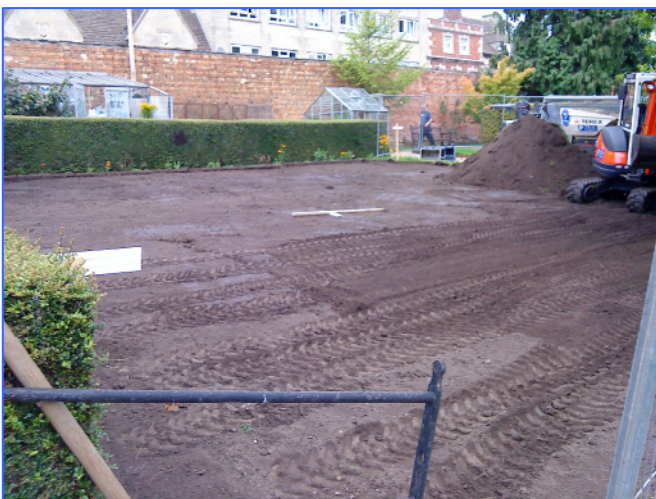
Plate 3: General view of the stripped area at the completion of groundworks. Looking north-east
