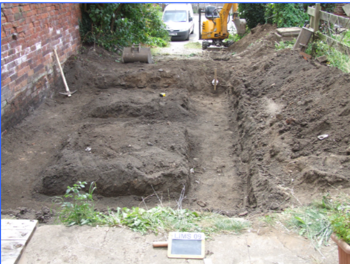
Plate 2: General view of the foundation trenches, looking south from the north end of the site.
