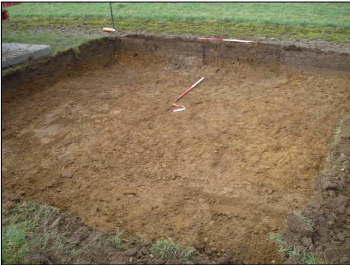
Plate 2: The excavation area on the site of the turbine base, looking south-west
