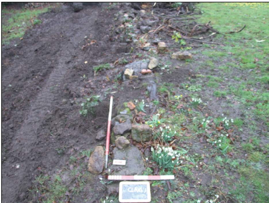
Plate 2: Collapsed wall spread 02 looking east
