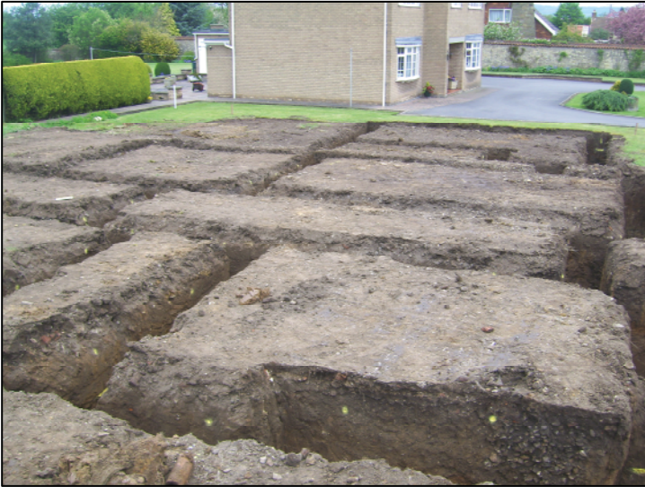
Plate 1: General view of the excavated footings, looking north. Note soakaway [07] in the bottom right-hand corner of the shot
