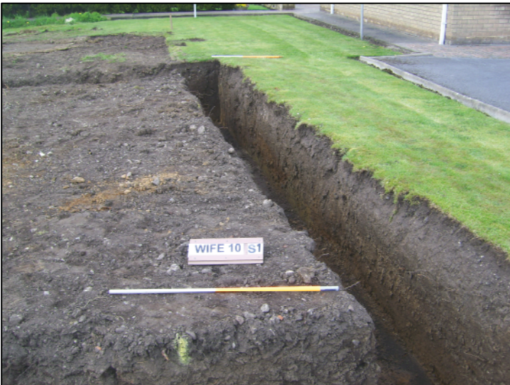
Plate 2: Detail of foundations along northern side of the site, looking north-west (section A-B)
