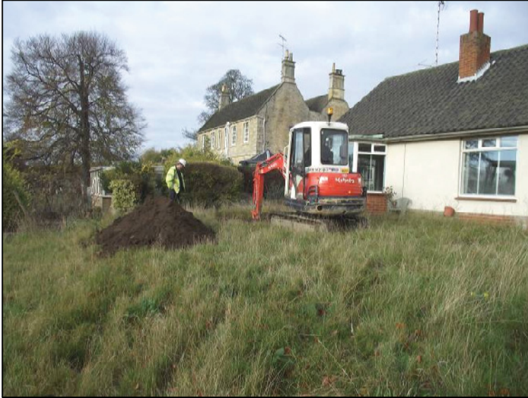
Plate 1: General view of the site at the commencement of the works, looking west-north-west
