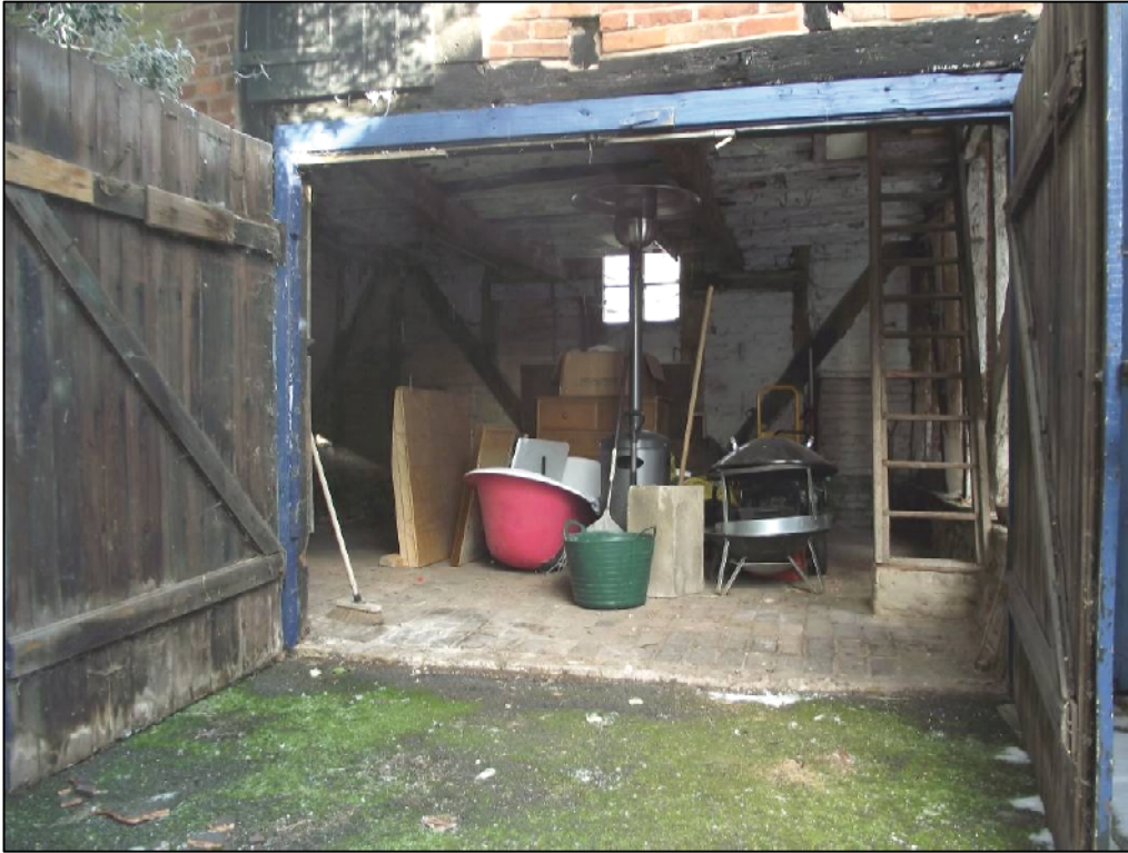
Plate 11 (Shot 14): General interior shot of the western bay of the building, looking north
