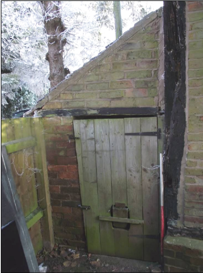
Plate 3 (Shot 6): Coal store on the south-west corner of the building. Looking north
