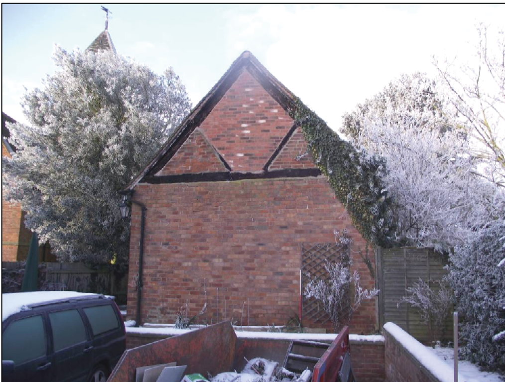
Plate 6 (Shot 3): General view of the east elevation of the later extension. Note the exposed roof structure and the modern brick repair. Looking west
