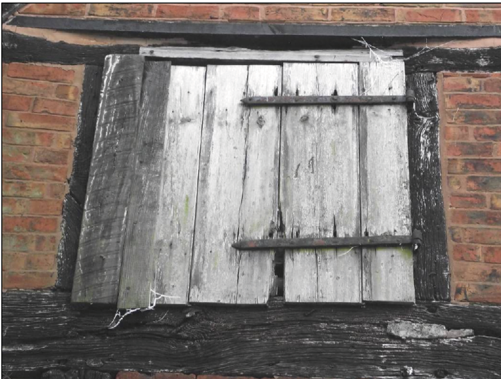
Plate 4 (Shot 8): Detail of pitching hole in west elevation, with replacement beam above. Looking east
