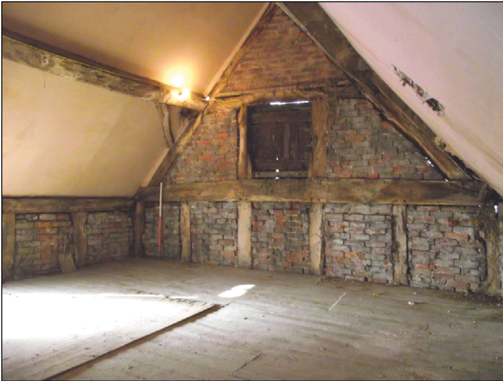
Plate 7 (Shot 15): Representative shot of the queenpost truss in the west gable. Looking west-south-west
