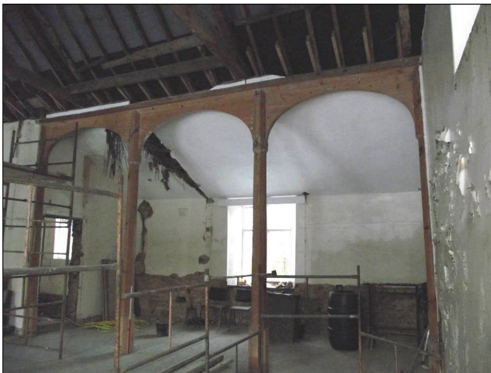
Plate 11 (Shot 25): Wooden arcade dividing the north-west corner of the chapel. Doorway to the left of shot leads to the kitchen. Looking west-south-west
