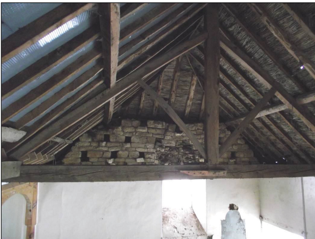
Plate 9 (Shot 20): Interior roof structure of the converted dovecote, also showing dove holes and the traces of a psalm plate to the right of the window, looking north
