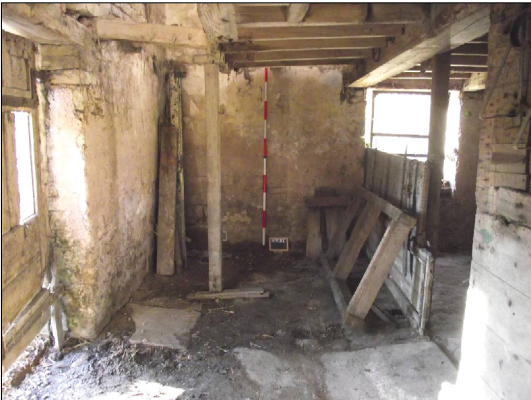
Plate 14 (Shot 29): General shot of the ground floor interior showing south and west elevations with plastered walls, remains of a stone slab floor, partition wall and above wooden support beams of the first floor. The opening in south-west corner of the ceiling would be used for hoisting up sacks of grain to second floor. Looking west
