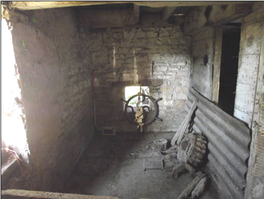
Plate 17 (Shot 32): General shot of north-west corner of the ground floor showing sluice wheel and wooden partition within cog house. Note the absence of plaster from the majority of the walls in this area. Note also the cog (stone nut) and other ephemera. Looking north
