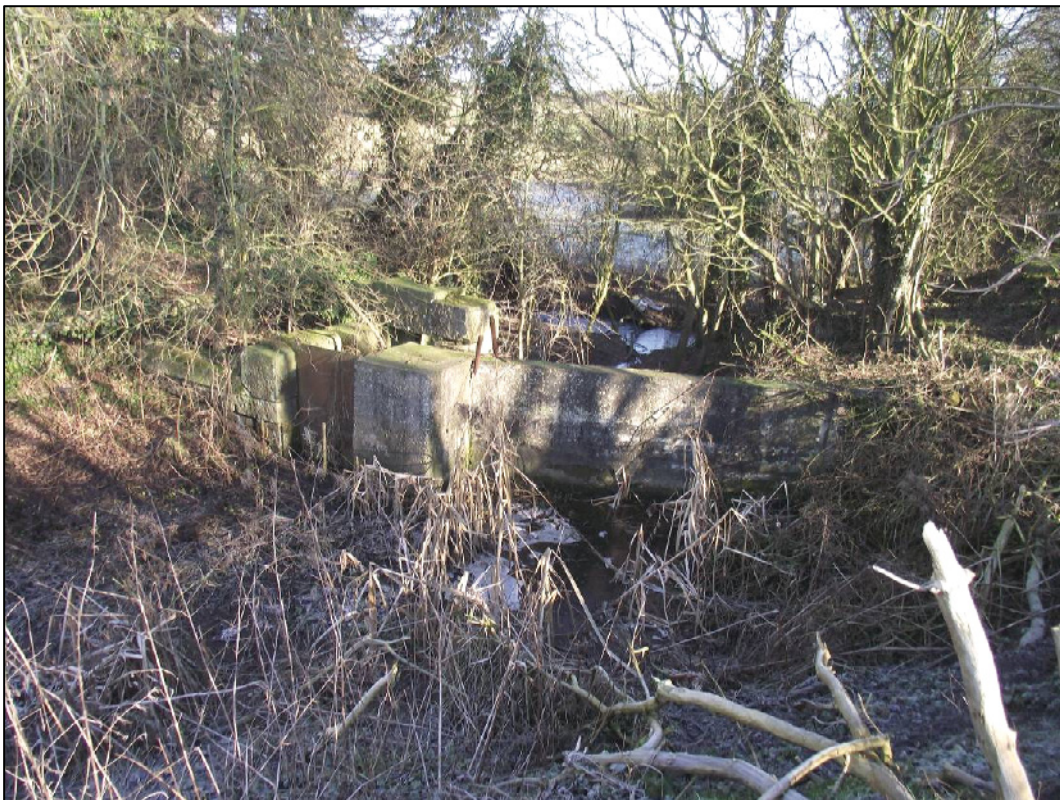
Plate 10 (Shot 19): Overgrown mill dam and weir west of the mill and mill race, looking east-north-east
