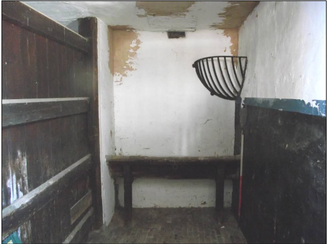
Plate 7 (Shot 10): Detail of stable with a feeding trough and a metal hayrack. Also notice the hatch from the hayloft above, looking south-west
