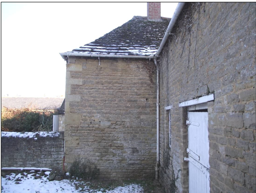
Plate 2 (Shot 3): South-east elevation of the tack room showing half-hipped roof. The brick chimney is a later addition. Looking north-west
