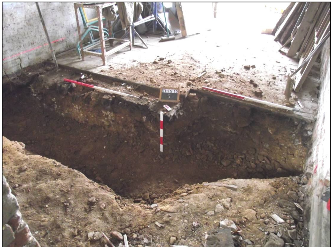
Plate 18: General shot of ground reduction inside the garage, showing south-west facing section, looking north-east
