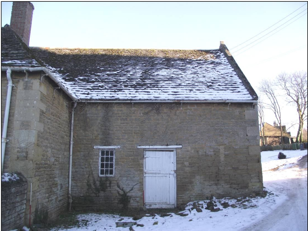
Plate 1 (Shot 1): South-west elevation of eastern range also showing the corner of the possible later extension to the left, looking north-east
